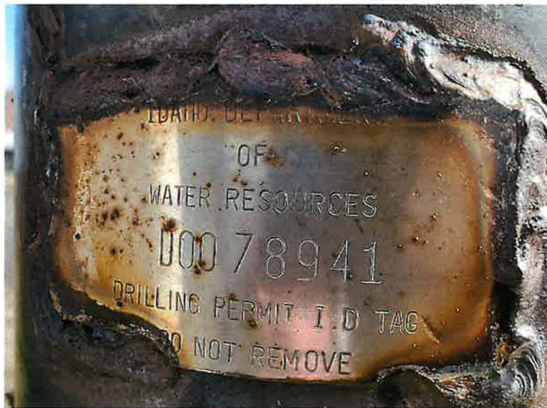
WELL, WELL METER AND WELL TAG D0078941
