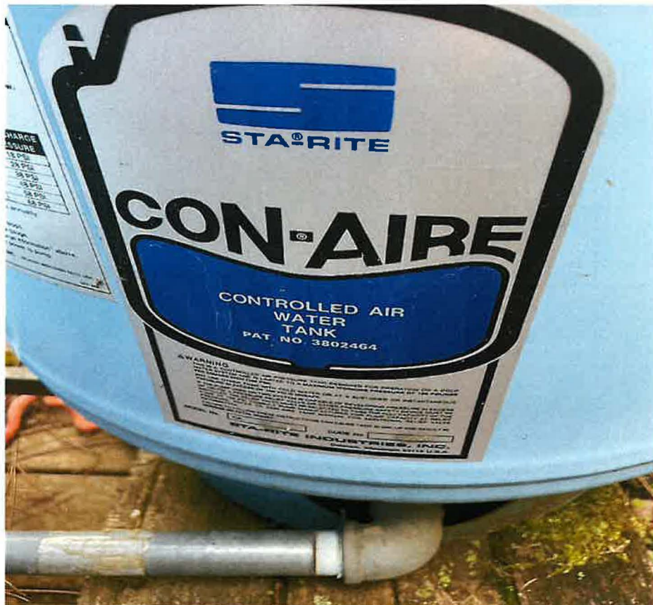
WATER SYSTEM COMPONENT – STA-RITE PRESSURE POT
