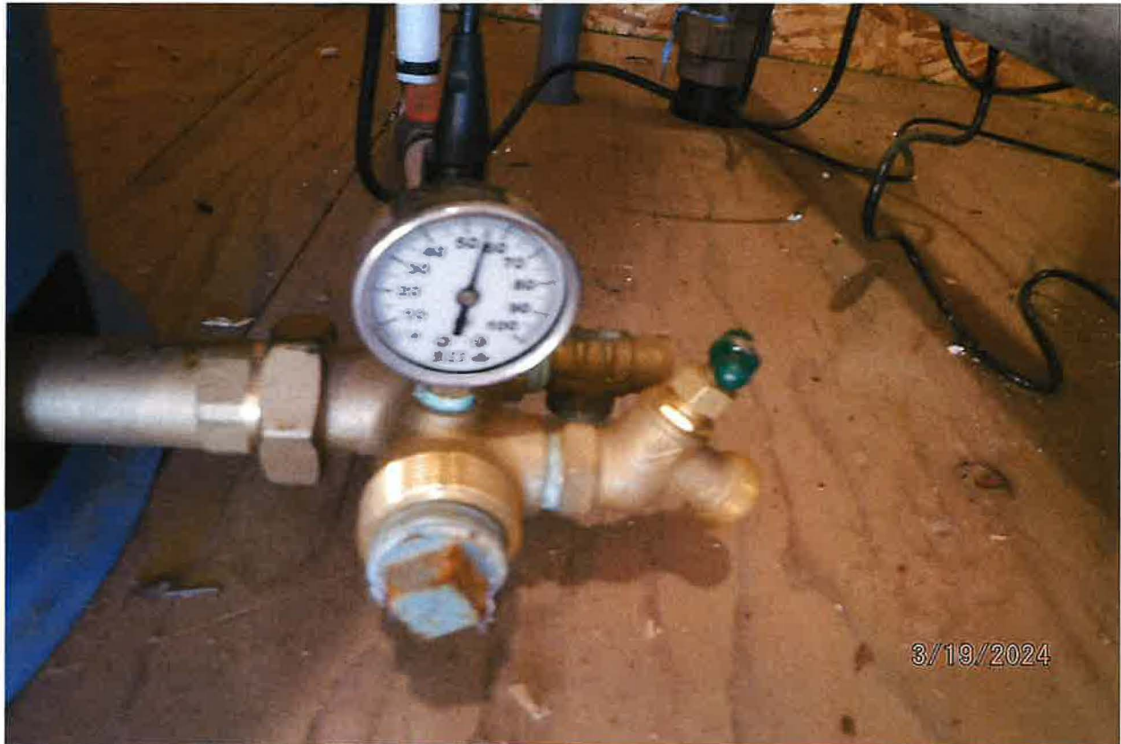
PRESSURE TANK INSTALLED ON SYSTEM HOLDS AT 55 PSI
