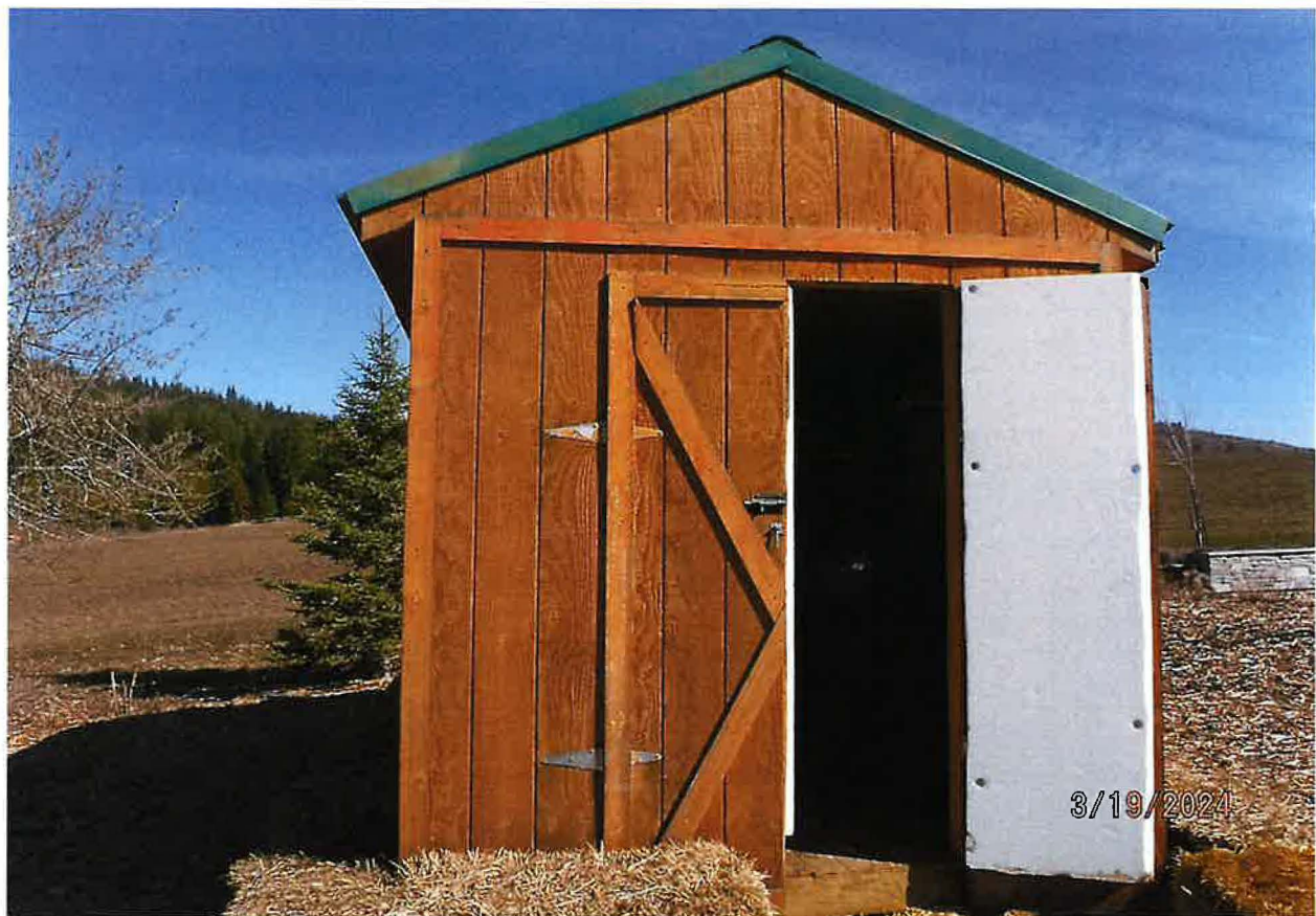
PUMP STATION – HOUSES CONTROLS FOR TWO SEPARATE WATER SYSTEMS (95-17566 & 95-17621)
