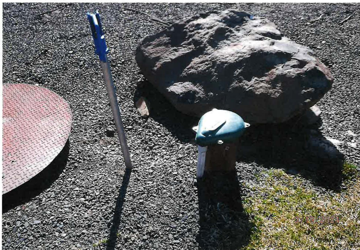
POD – GROUNDWATER WELL – NO D-TAG ON CASING
