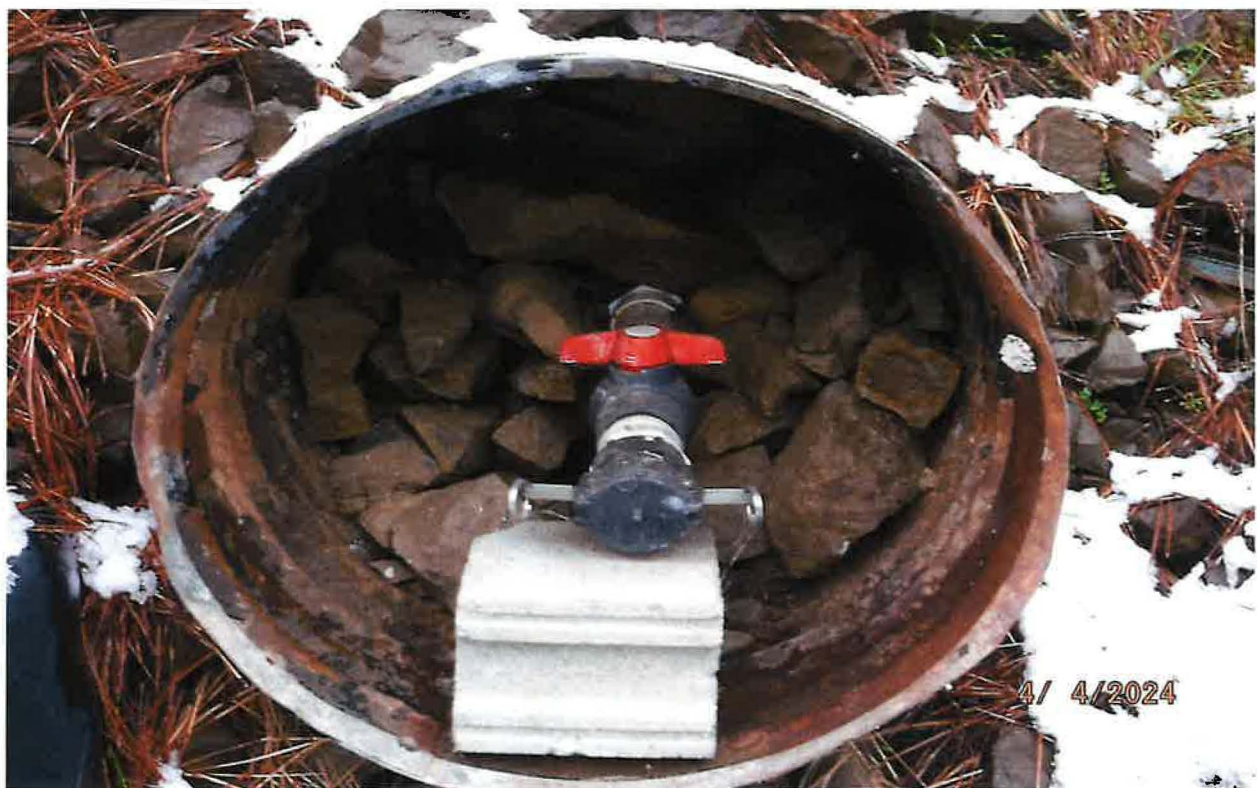
FIRE PROTECTION FROM STORAGE FIRE HOSE CONNECTION VALVE WITH MANUAL SHUTOFF VAVLE
