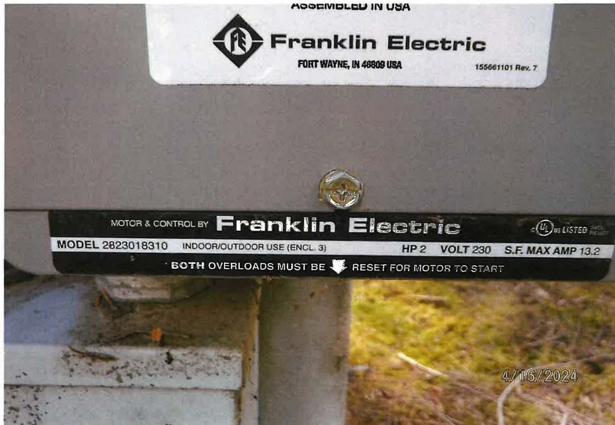
2 HP FRANKLIN ELECTRIC PUMP MOTOR INSTALLED IN WELL 96-95-N-0210
