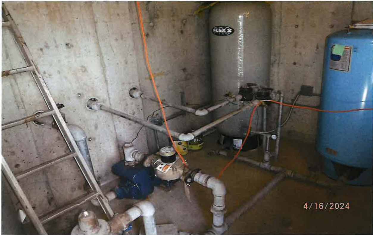
WATER CONVEYANCE SYSTEM – TOP PIPES 1EA FROM RESPECTIVE WELL WITH FLOW METERS TO STORAGE (LEFT CENTER OF IMAGE) AND 1EA PIPE TO 5 HP CENTRIFUGAL PIPE WITH FLOW METER FROM STORAGE RESERVOIR
