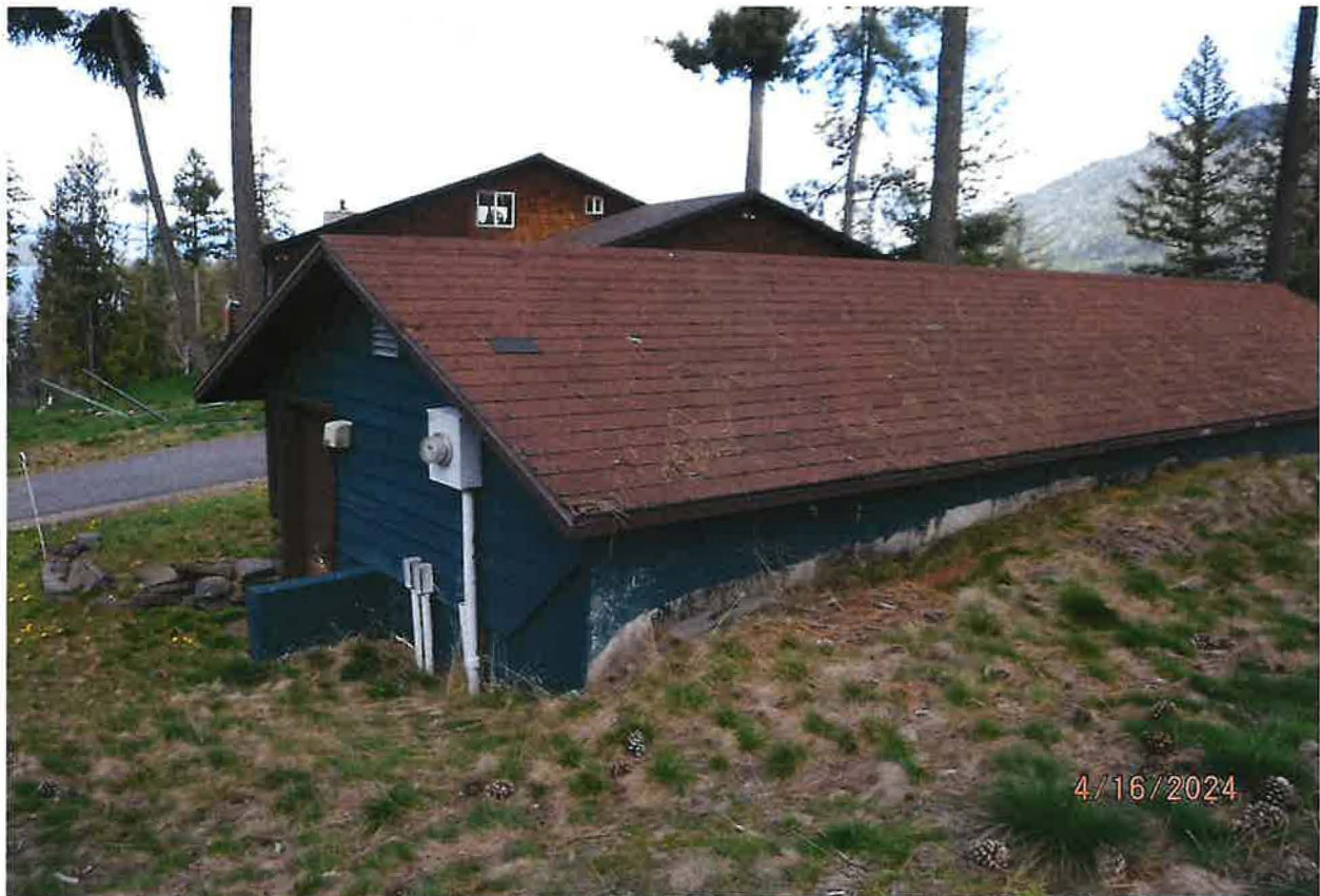
PUMP STATION & 16,000+ GALLON COMMUNITY STORAGE RESERVOIR
