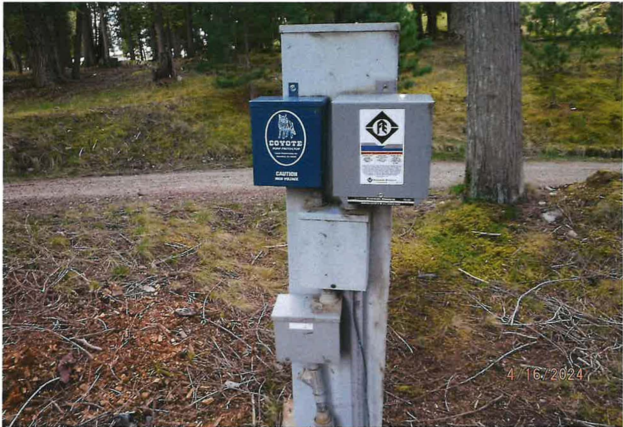
WELL 96-95-N-0210 ELECTRIC CONTROL PANEL – CO-LOCATED WITH WELL
