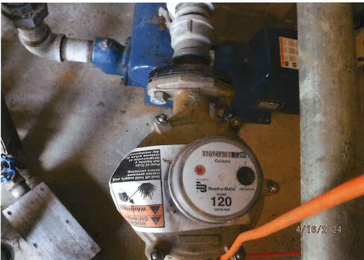
READ-O-MATIC MODEL 120 FLANGED VELOCITY STYLE FLOW METER – USED TO RECORD VOLUMETRIC DATA FROM THE COMMUNITY STORAGE RESERVOIR
