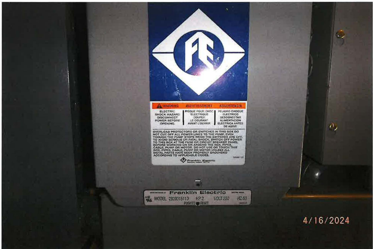
FRANKLIN ELECTRIC 2 HP PUMP MOTOR INSTALLED IN WELL 96-95-N-0302 (RELAY CONTROL PANEL LOCATED IN PUMP STATION – CO-LOCATED WITH 'HIGH' WELL)
