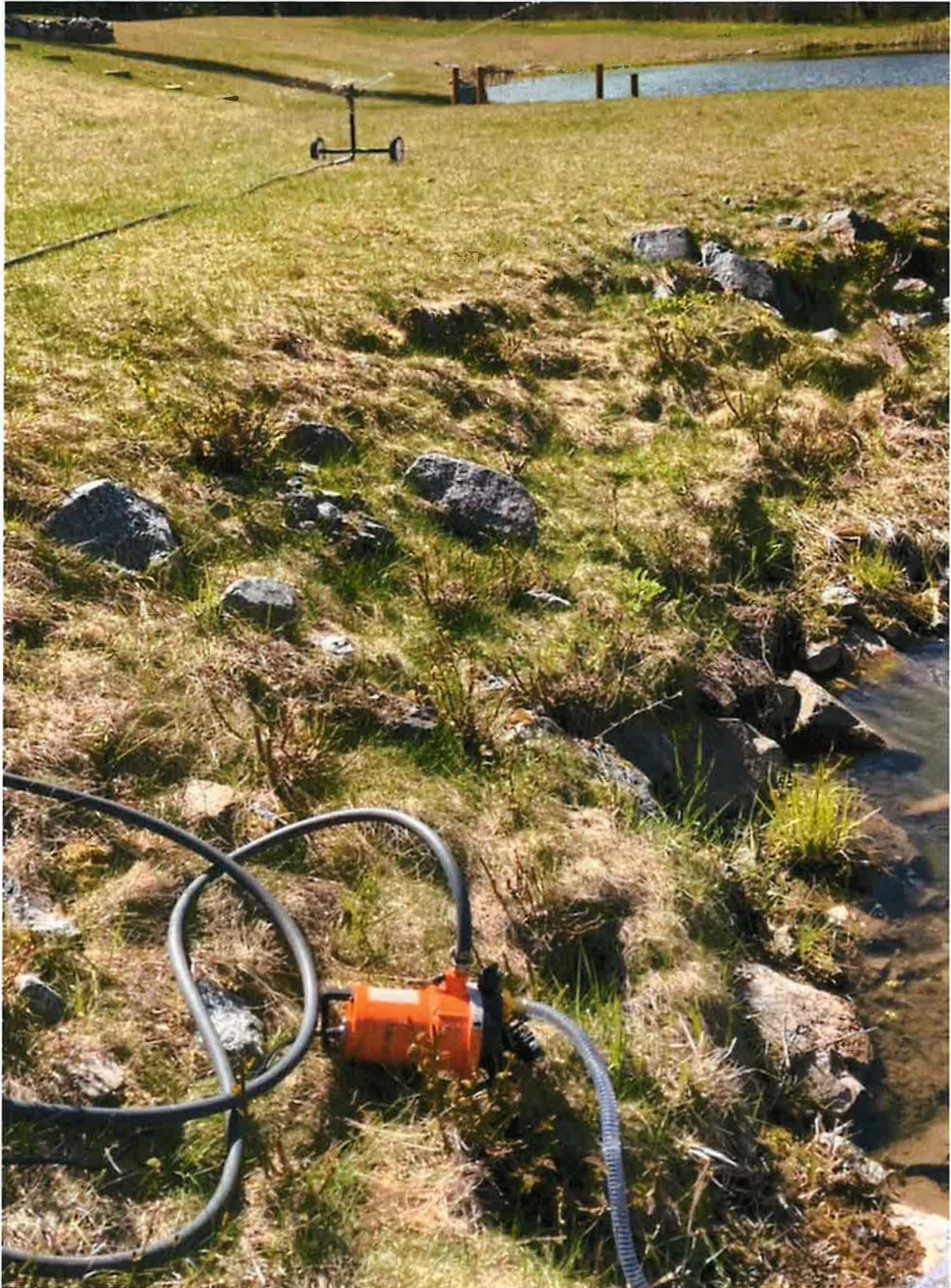
IRRIGATION POU - PORTABLE ELECTRIC PUMP WITH FLEXIBLE SCREENED INTAKE & HOSE TO SPRINKLER
