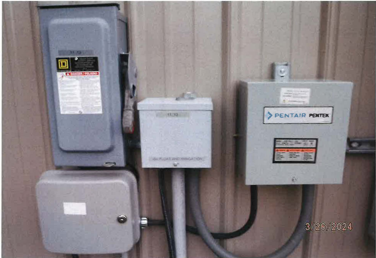
STORAGE CISTERN PUMP CONTROL LOCATED ON BACK OF BARN
