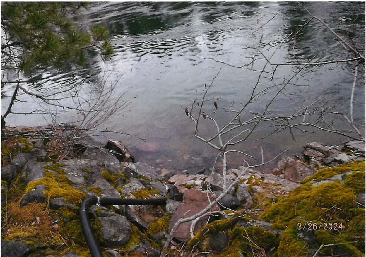
POD – SCREENED FLEXIBLE PIPE FROM SPOKANE RIVER TO DIVERTING PUMP
