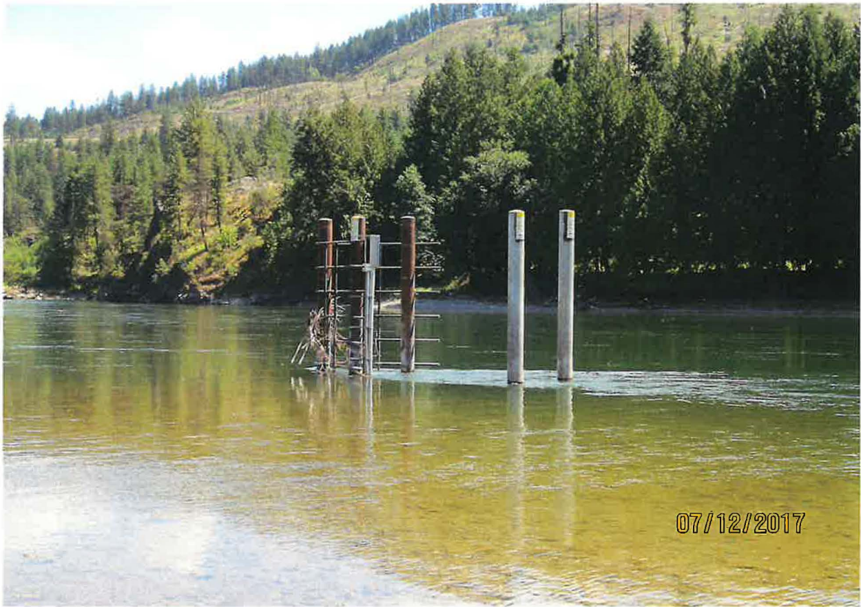
POD – KOOTENAI RIVER INTAKE WORKS
