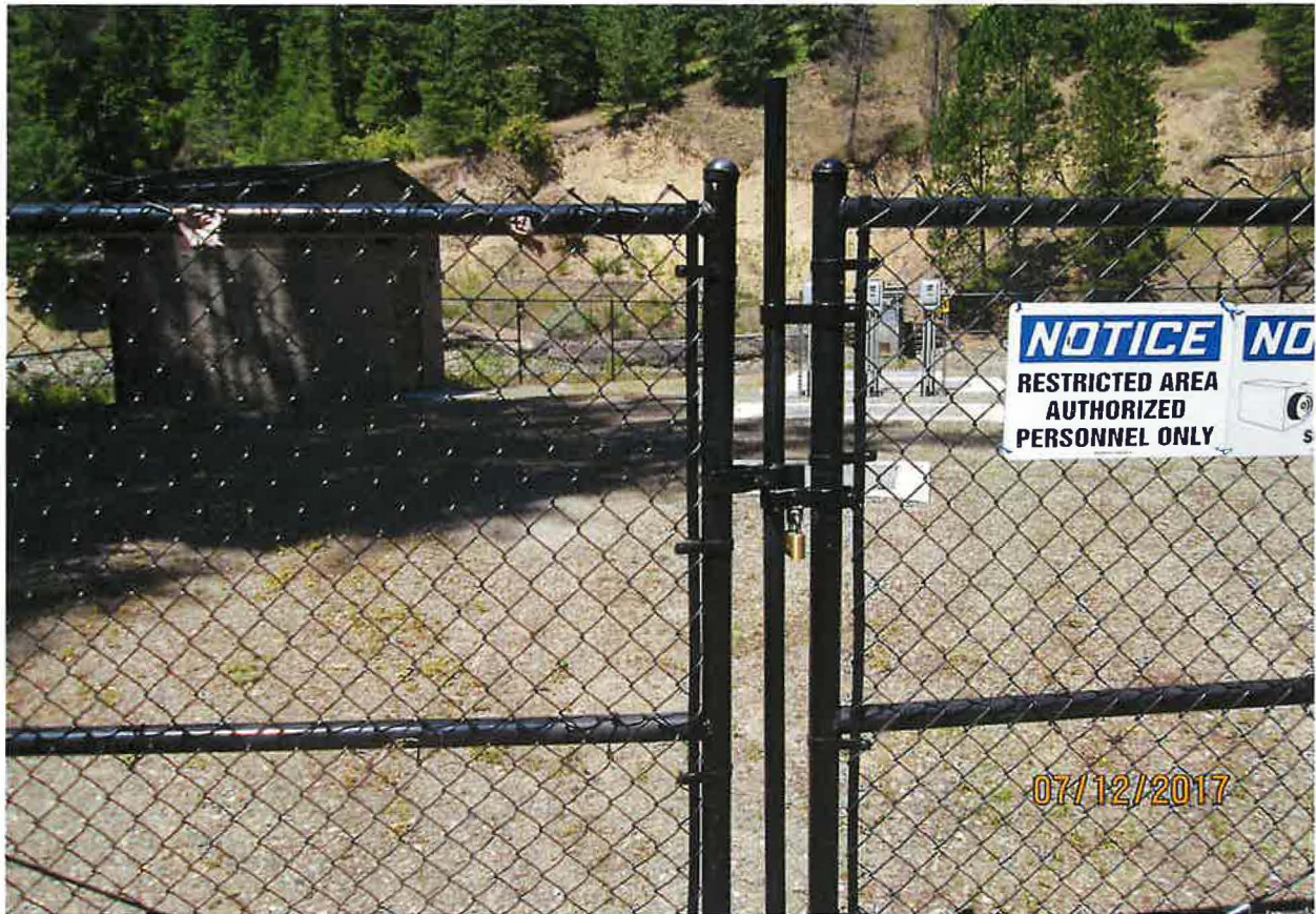
MOYIE RIVER CONVEYANCE SYSTEM PUMP STATION
