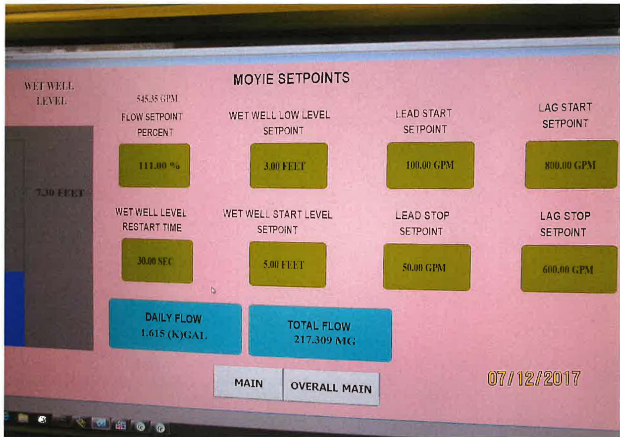
HATCHERY SCADA SYSTEM – MOYIE SETPOINTS
