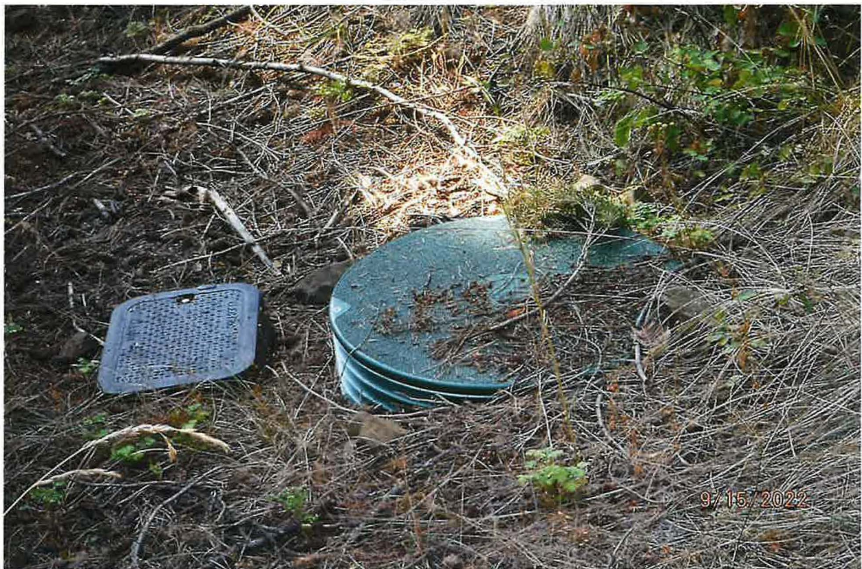
STORAGE CISTERN – SURFACE WATER PUMPED TO THIS CISTERN WHERE IT CO-MINGLES WITH A SEPARATE WELL WATER SOURCE PRIOR TO DISTRIBUTION TO WATER USES
