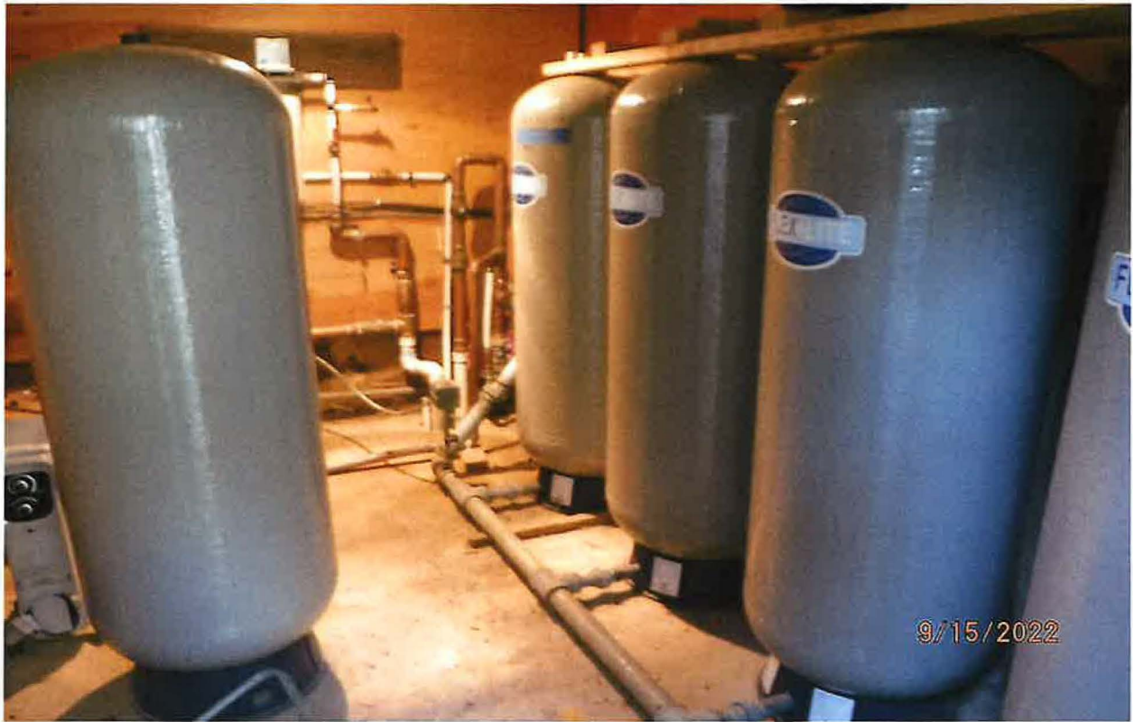
WATER SYSTEM COMPONENTS – MULTIPLE PRESSURE TANKS USED TO FACILITATE DOMESTIC & IRRIGATION USE IN SUBDIVISION.
