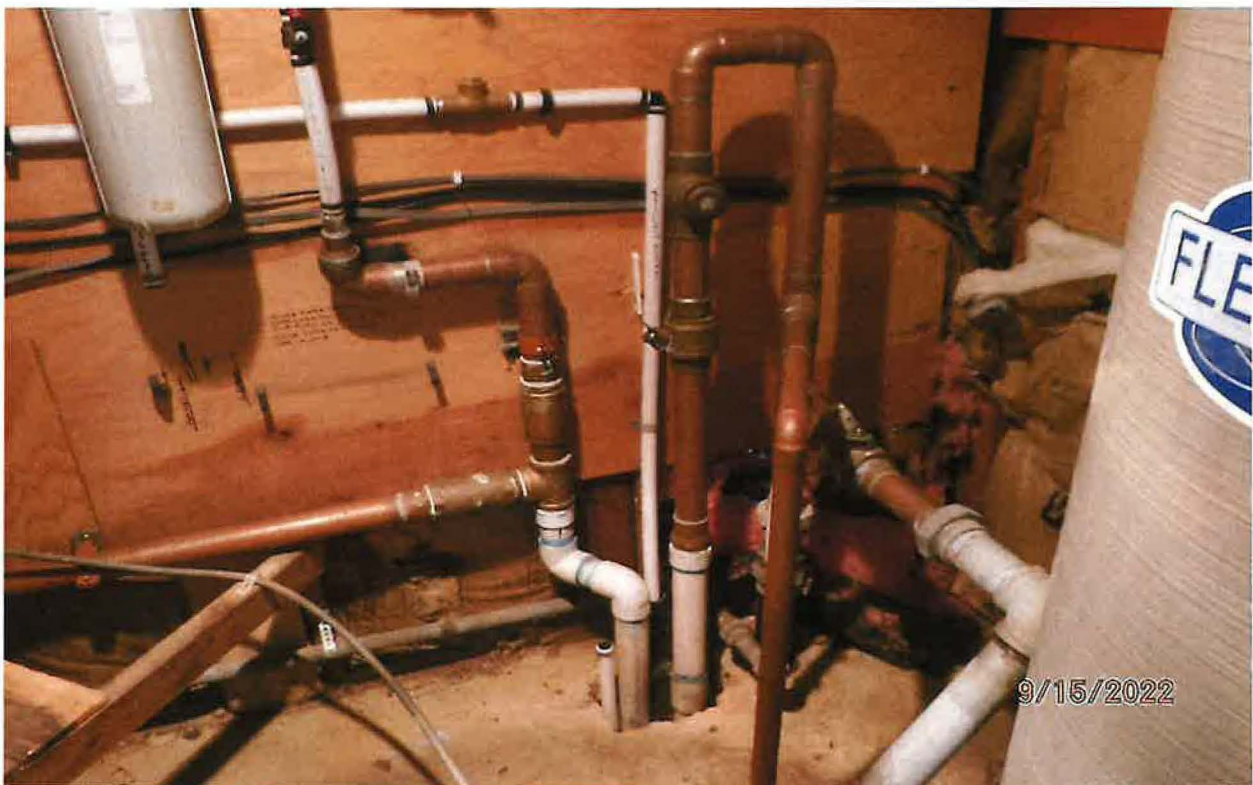
CO-MINGLED WATER CONVEYANCE SYSTEM – GROUNDWATER WELL PUMP HOUSE AND COMBINED USE SURFACE WATER SYSTEM
