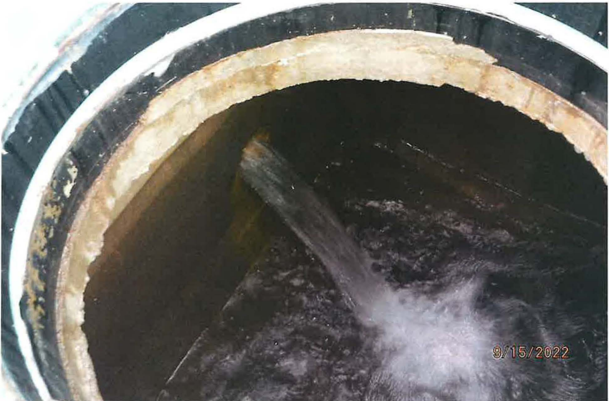
UNABLE TO PERFORM FLOW MEASUREMENT DUE TO INADEQUATE PIPE REQUIREMENTS – OBSERVED FLOW INTO CISTERN FROM 2 HP SURFACE WATER PUMP
