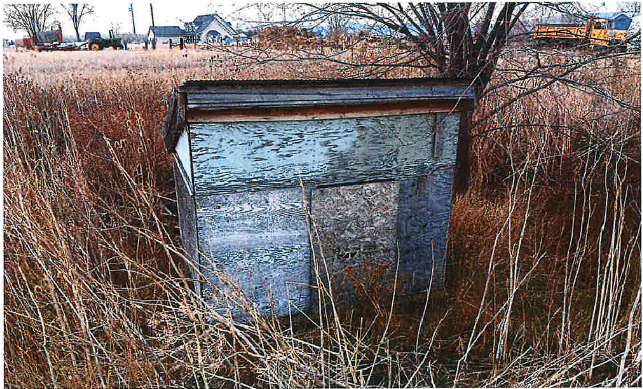
Low Water Pump House (taken 11/22/24)
