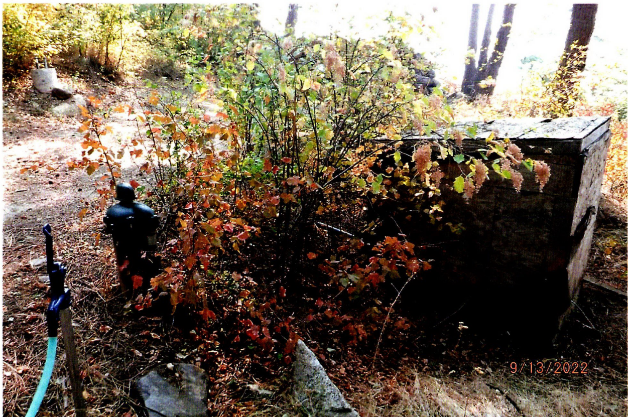
WOODEN PUMP STATION NEXT TO WELL
