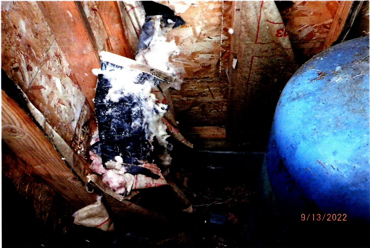
INTERIOR PUMP STATION
