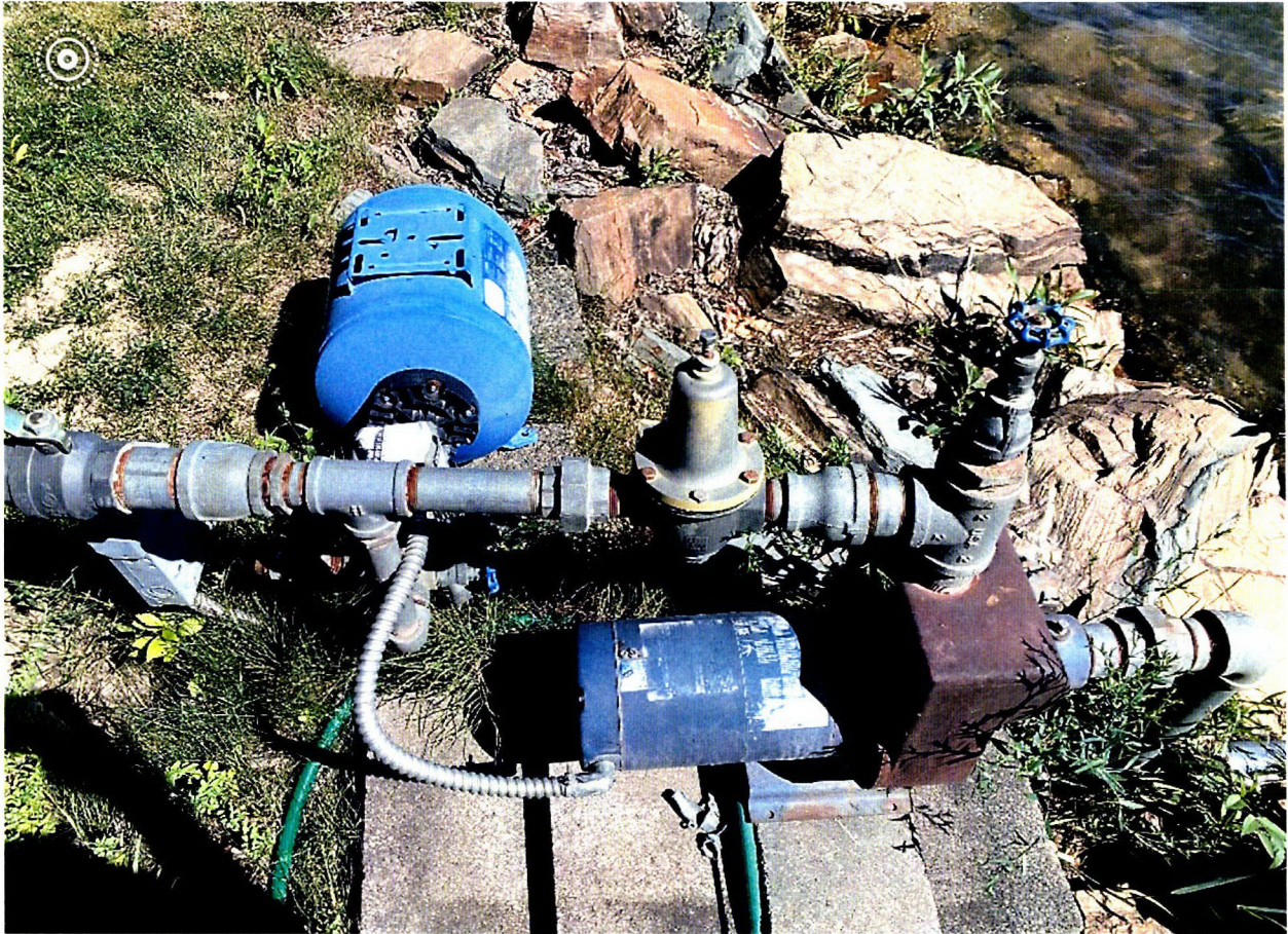
Figure 3: 2.5 HP pump with pressure tank. 2 inch line to pump
