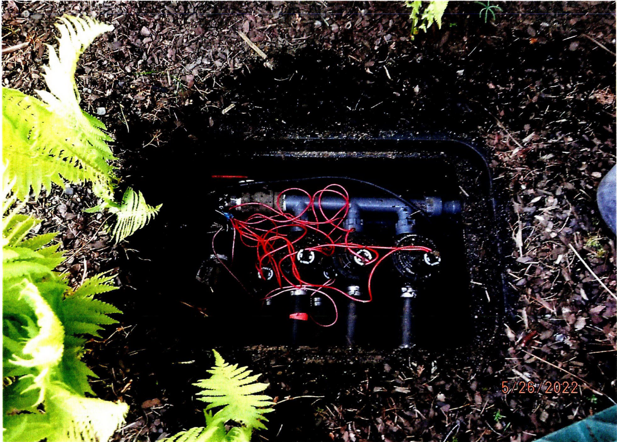
IRRIGATION CONTROL BOX FOR UPPER 5 ZONES
