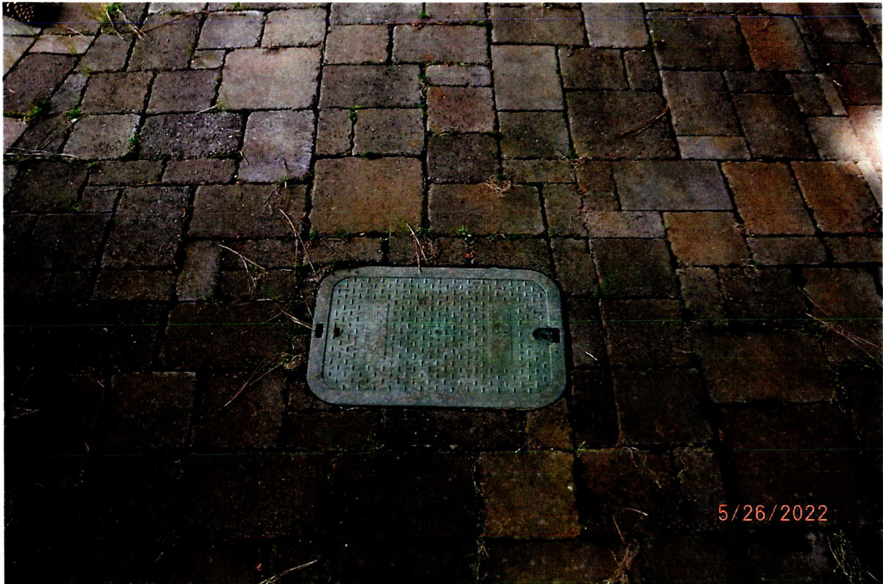
MAIN WATER LINE SHUTOFF VALVE BOX – LOCATED NE CORNER OF MAIN RESIDENCE
