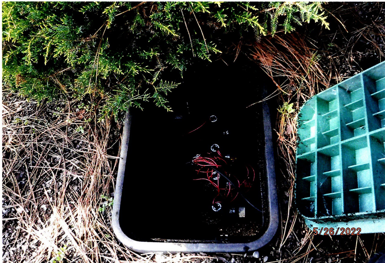
IRRIGATION CONTROL BOX FOR LOWER 4EA ZONES
