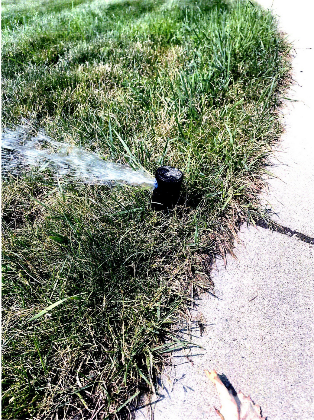
Photo 5- Pop up sprinklers used for system with drip lines.
