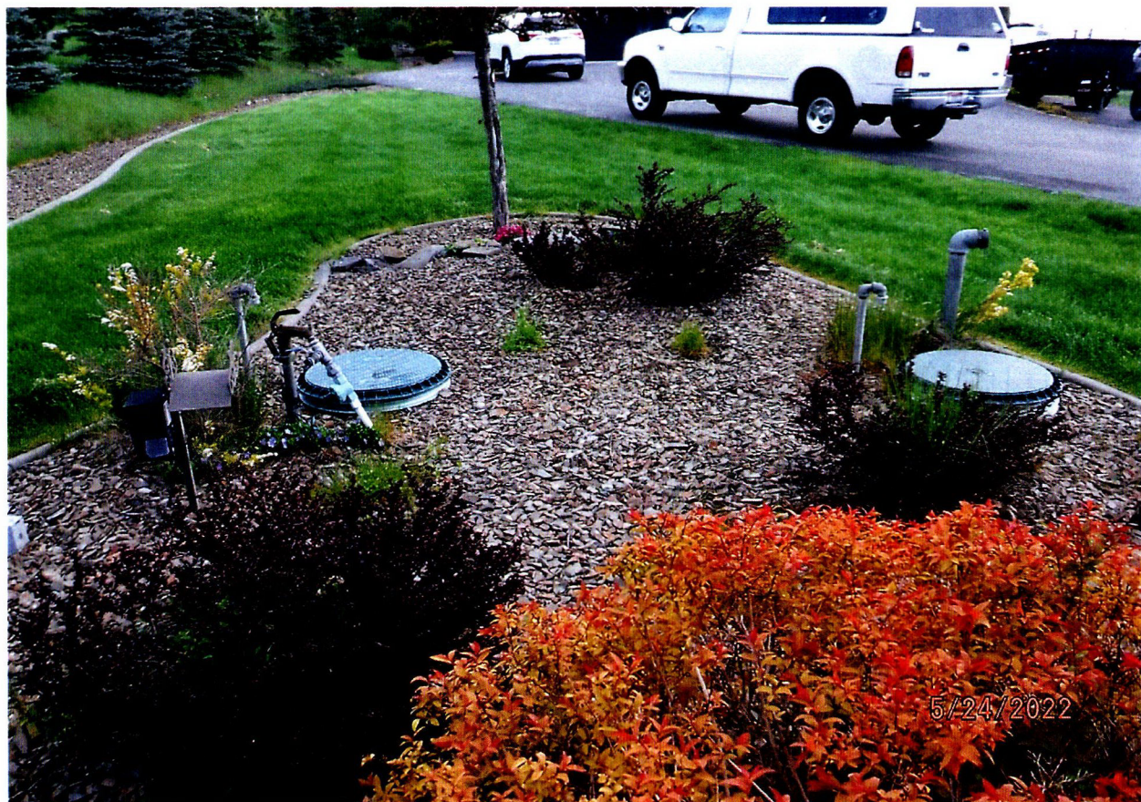
WATER FROM WELL DIVERTS DIRECTLY TO 2EA 3,000 GAL STORAGE TANKS BEFORE USE
