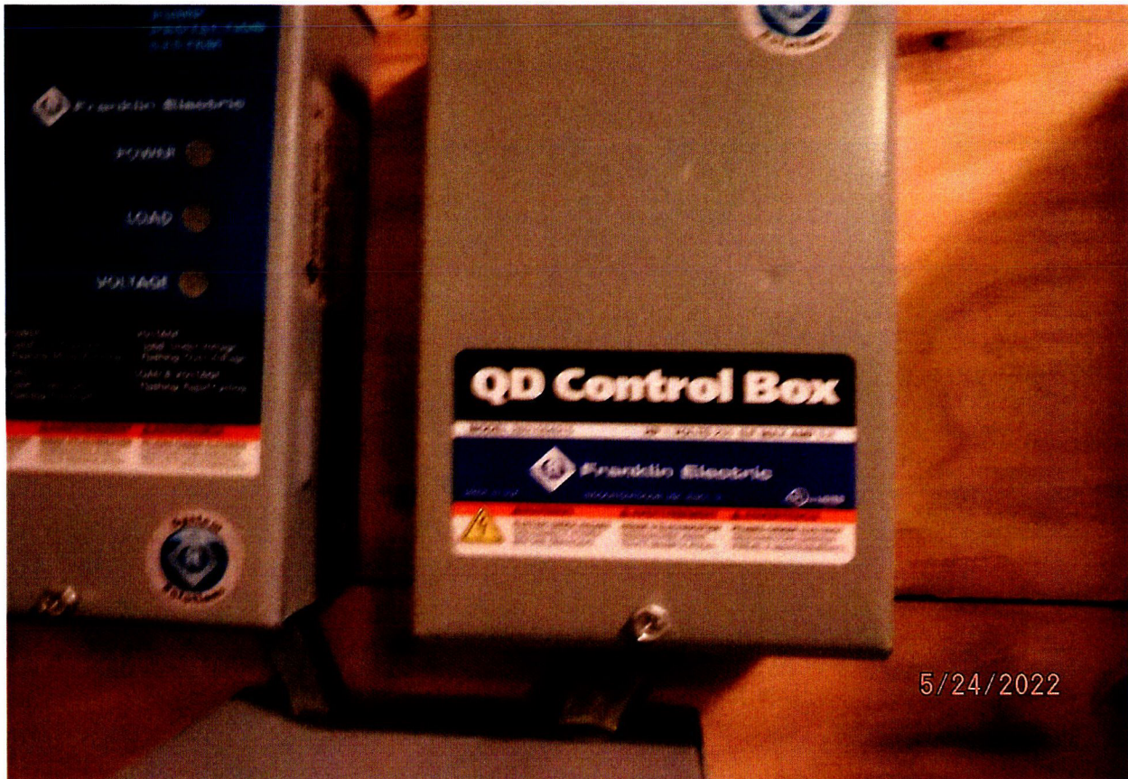
1 HP FRANKLIN PUMP MOTOR (2EA) INSTALLED IN STORAGE TANKS
