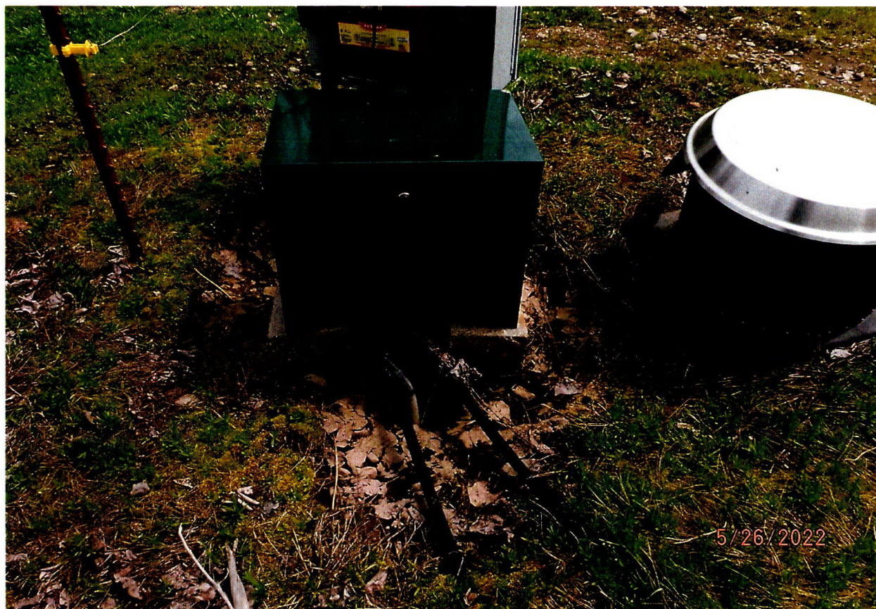
AERATORS (2EA) CONTROL UNIT
