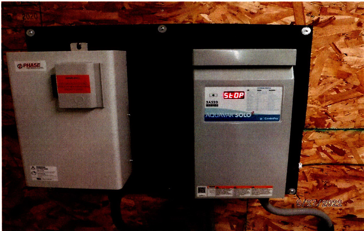
GOULDS 1.5 HP PUMP MOTOR INSTALLED IN WELL – MODEL 7GS15412
