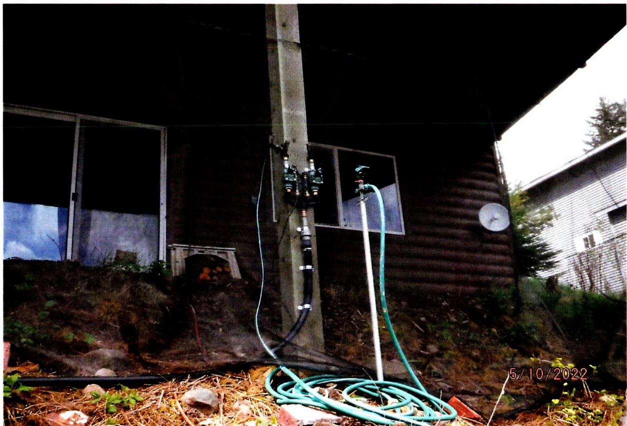
IRRIGATION SYSTEM RISER PIPE WITH SPRINKLER
