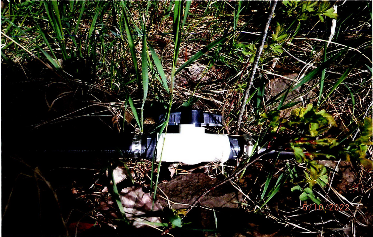
MANUAL SHUTOFF BALL VALVE IN-LINE AT POD
