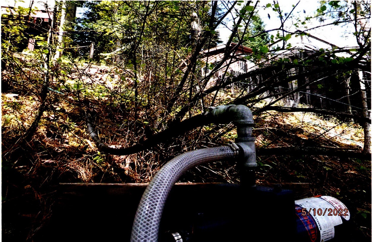
MAIN IRRIGATION POLY PIPE ROUTES UP-HILL TO IRRIGATION RISER PIPES
