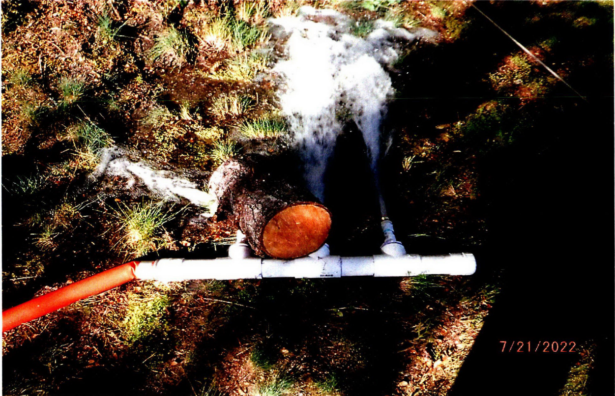
IRRIGATION SPLITTER WITH 3EA HOSE CONNECTIONS
