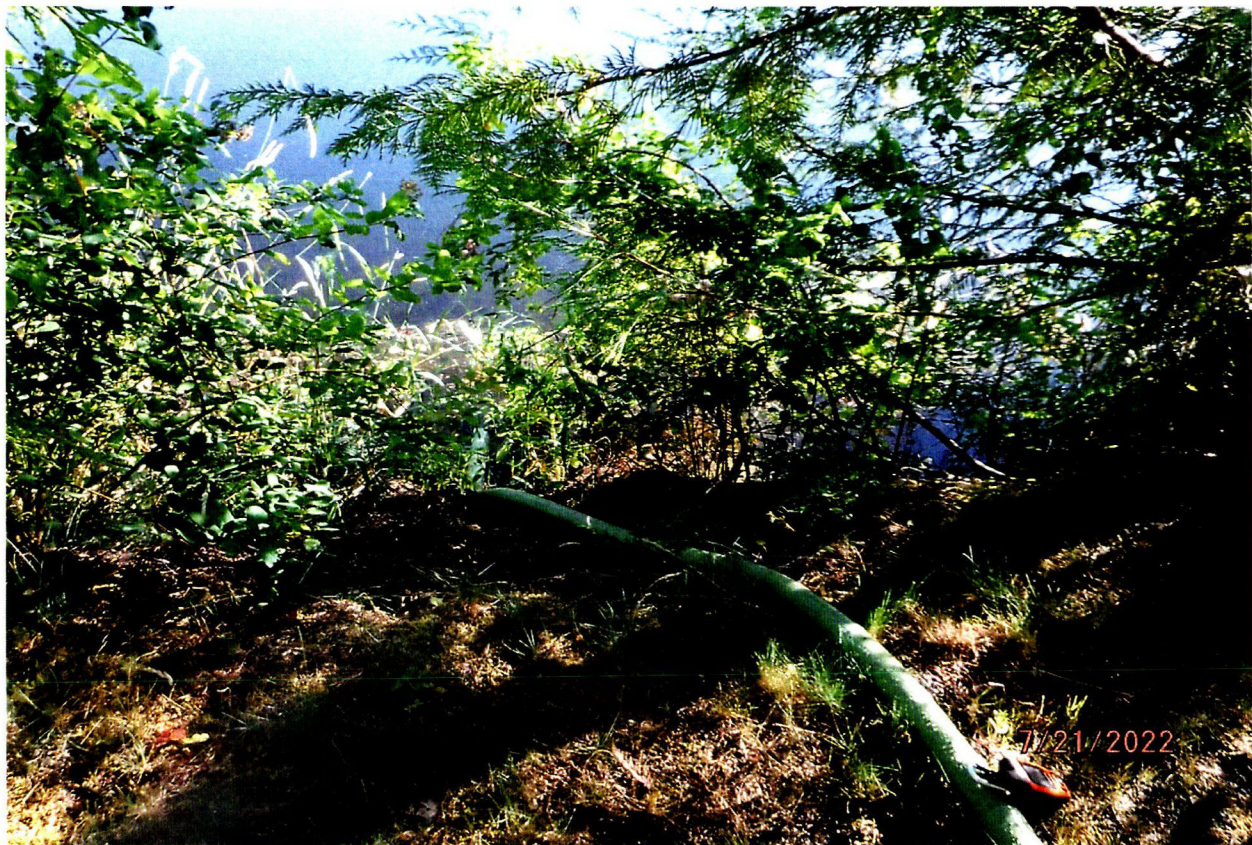
POD – SCREENED INTAKE PIPE TO WATER TRANSFER PUMP
