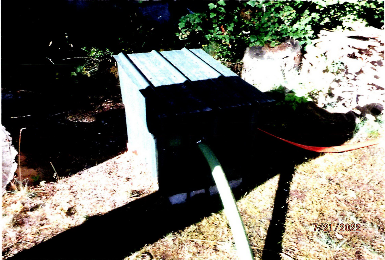
WATER TRANSFER PUMP DOG HOUSE
