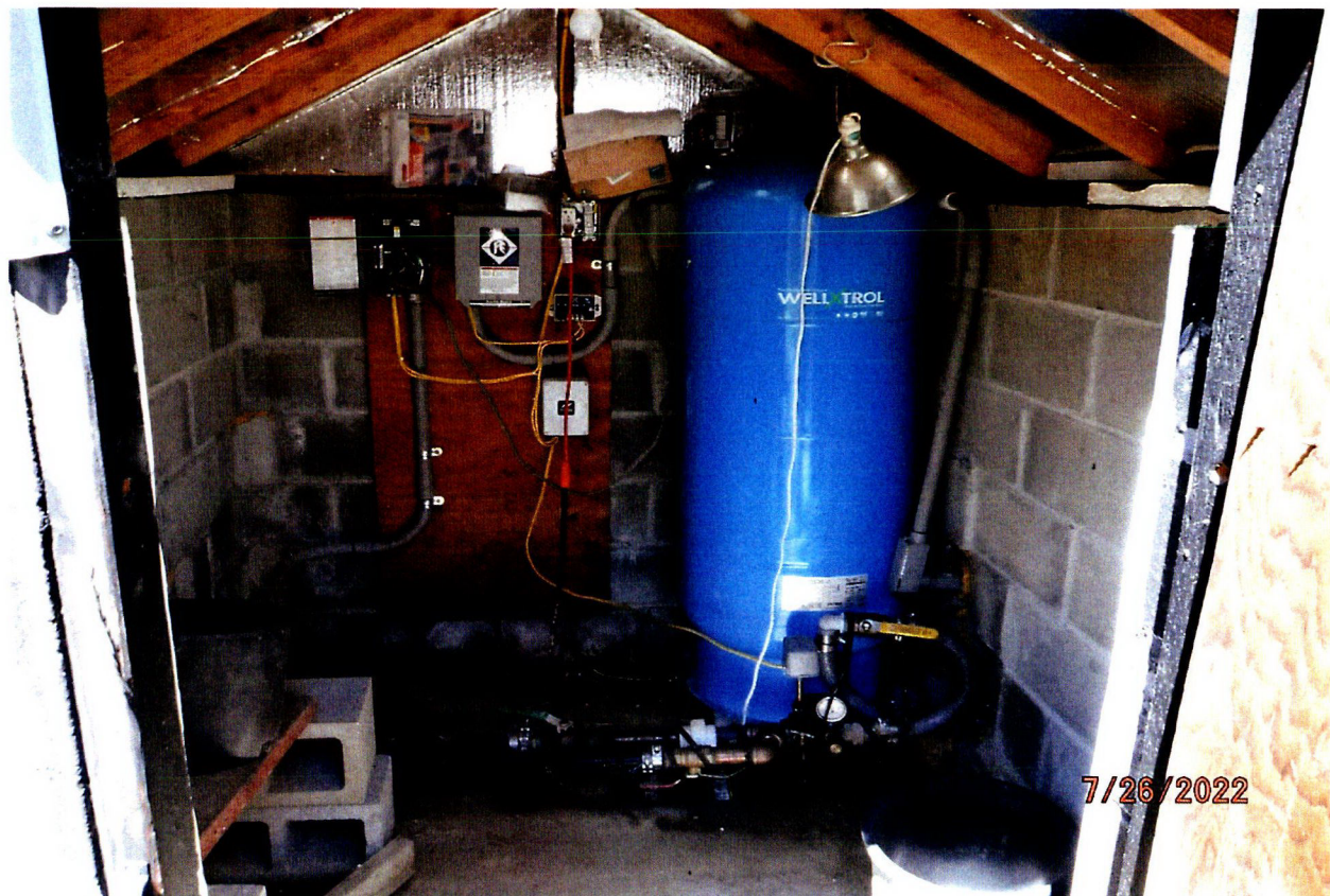
PUMP HOUSE – WATER DIVERTING WORKS
