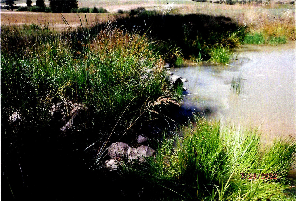
ROCKED OVERFLOW CHANNEL ALLOWS WATER TO FLOW DOWNGRADE FROM POND
