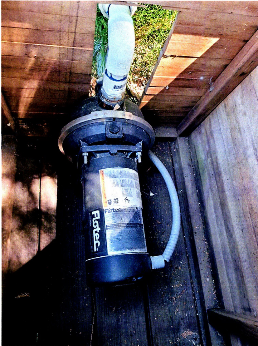
Figure 3- Photo of the Flotec 1 ½ Hp pump in the “doghouse” beside the southeast corner of the dock
