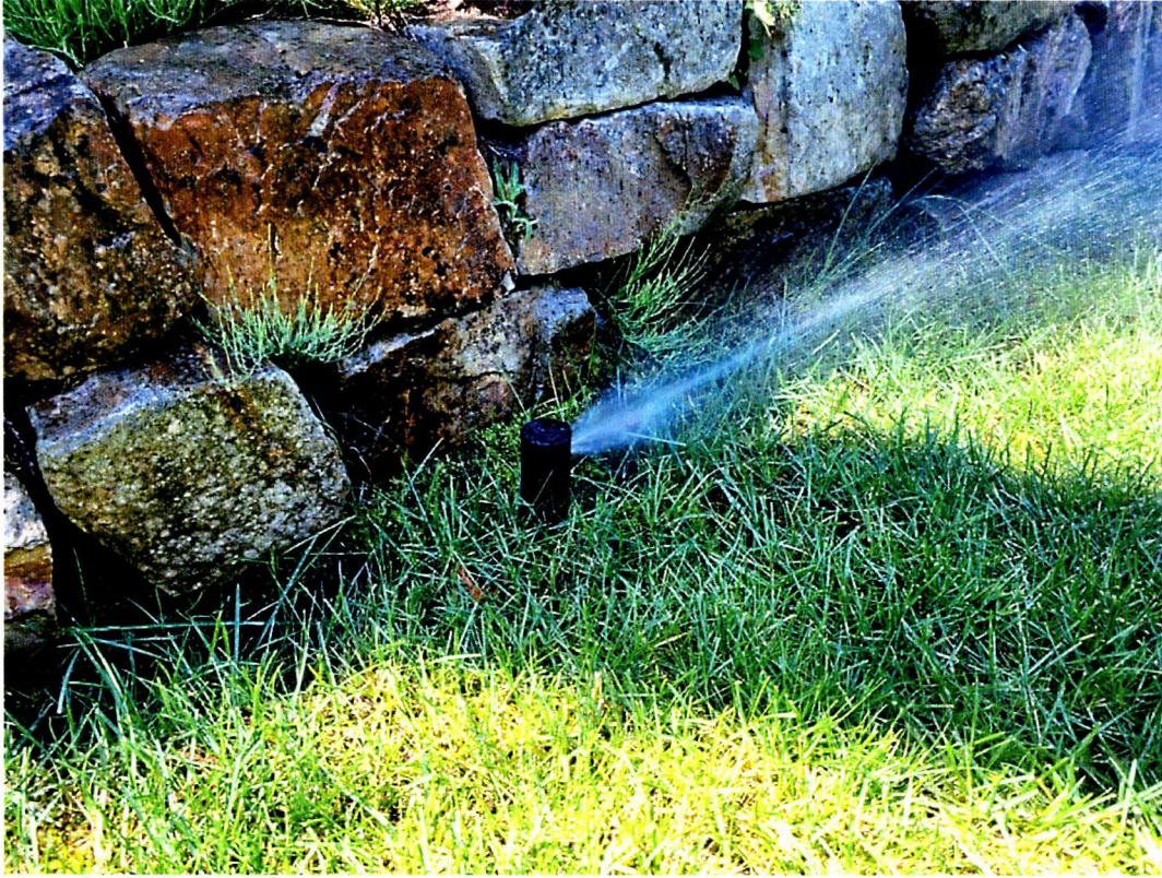
Figure 6- Photo of one of the popup sprinklers used throughout the irrigated areas.
