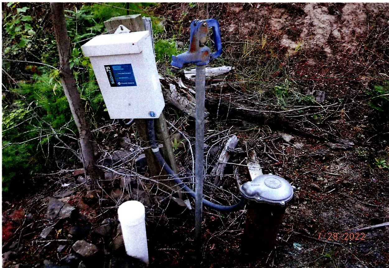
POD – GROUNDWATER WELL
