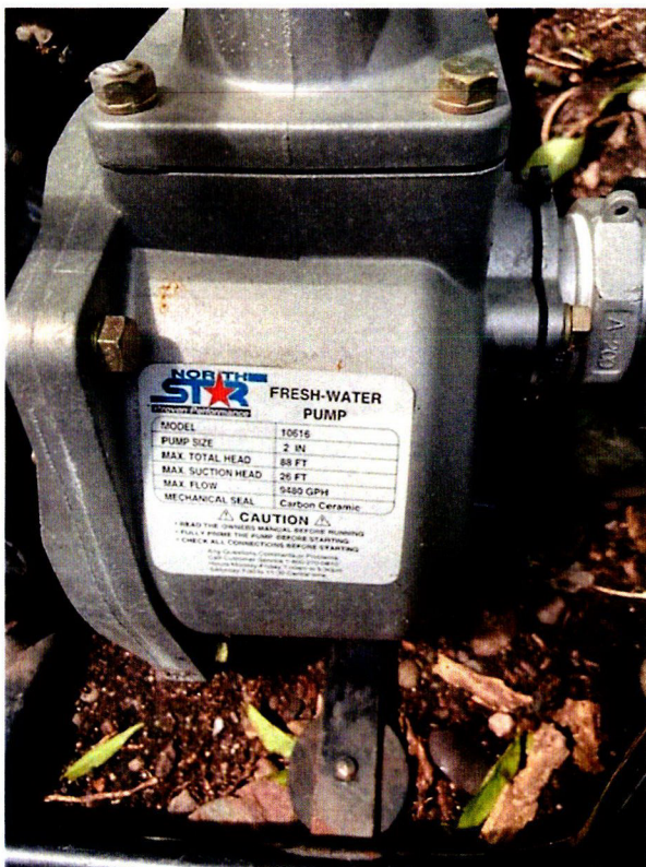
Specification plate for pump.
