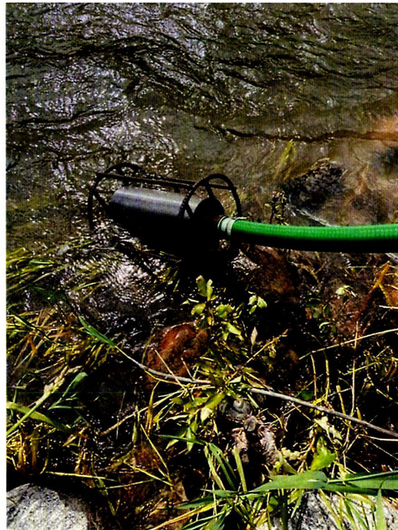
Fish screen on pump intake.
