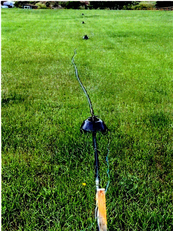
North sprinkler line.
