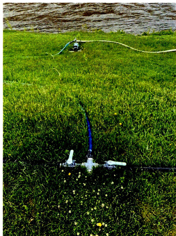
Manifold divides water between N & S lines.
