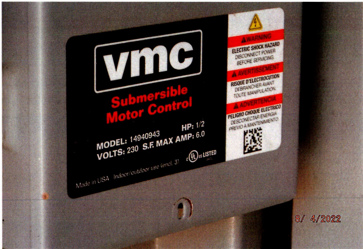
½ HP PUMP MOTOR INSTALLED IN DIVERTING WORKS
