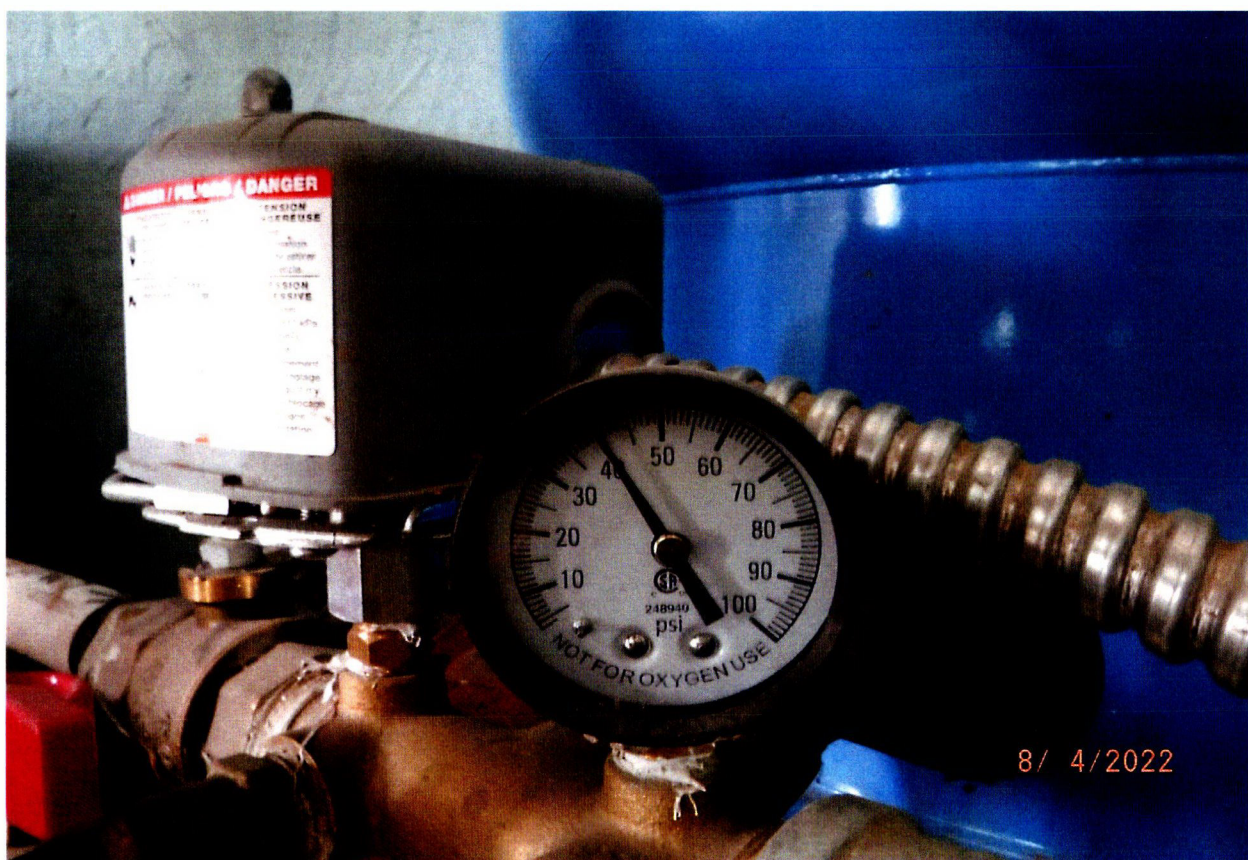
40 PSI OPERATING PRESSURE AT PRESSURE TANK
