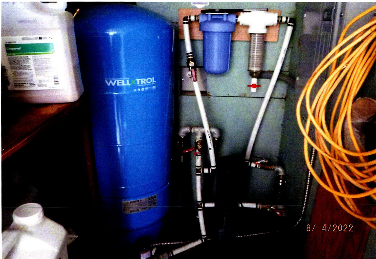
SPRING WATER PUMPED TO 4 FROST FREE HYDRANTS FOR STOCKWATER USE
