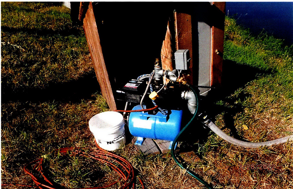
5 GAL BUCKET MEASUREMENT TAKEN FROM HOSE BIB CONNECTION AT POD
