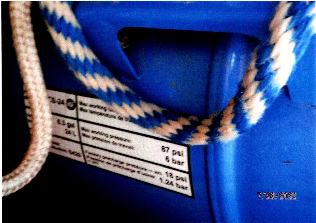
6.3 GAL PRESSURE POT WORKING AS PART OF THE TRANSFER PUMP UNIT
