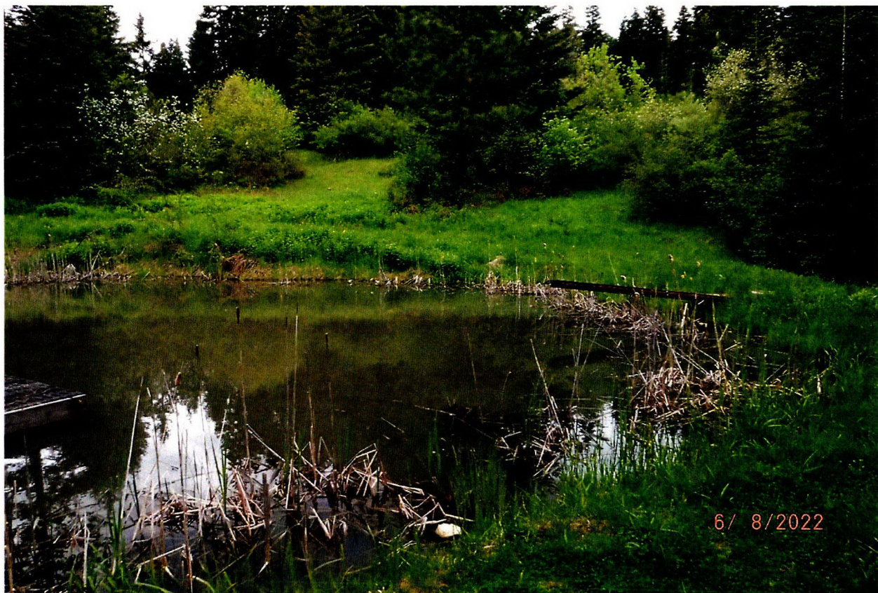
STORAGE POND DAM, NO OVERFLOW DEVICE CONSTRUCTED FOR POND
