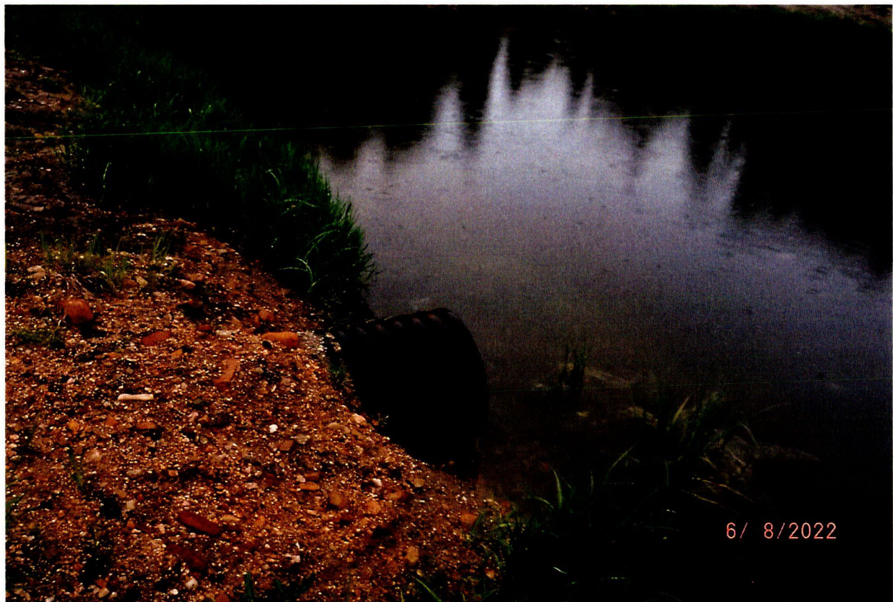
PLASTIC STORM PIPE OVERFLOW DISCHARGE CENTER MASS OF POND DAM
