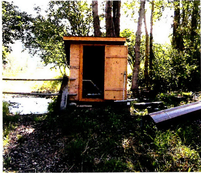
Figure 11 POU showing Turbine inside Enclosure
