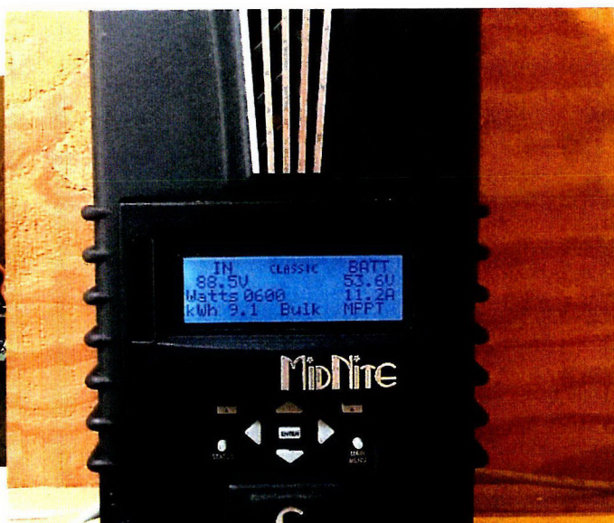
Figure 15 Control Panel for the Batteries & Hydropower Systems
