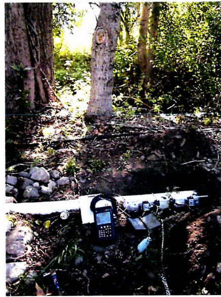
Figure 13 Field Measurement on the 6" Penstock
