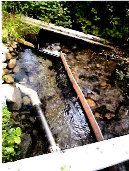
Figure 6 POD Showing Fish Screen and Diversion Structure in Pioneer Creek
