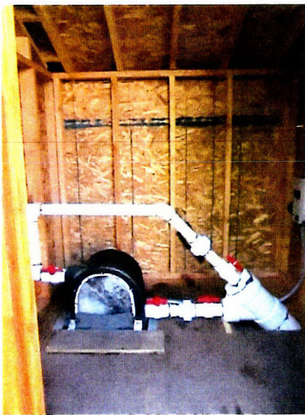
Figure 12 Penstock Penetrating Through Enclosure floor & 4" Pipes leading to 2 Nozzle Locations on the Turbine
