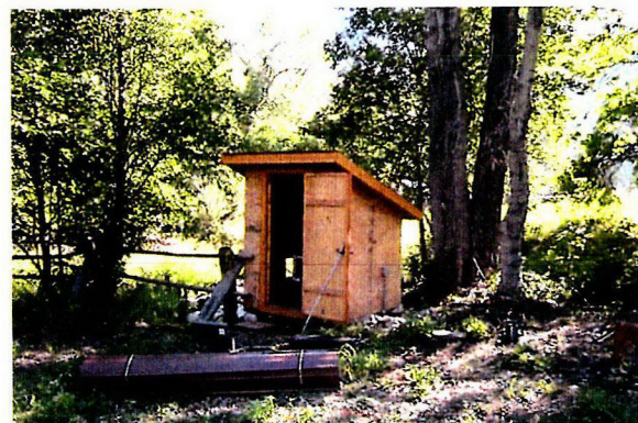
Figure 9 POU for Turbine Housed in a Wood Enclosure
