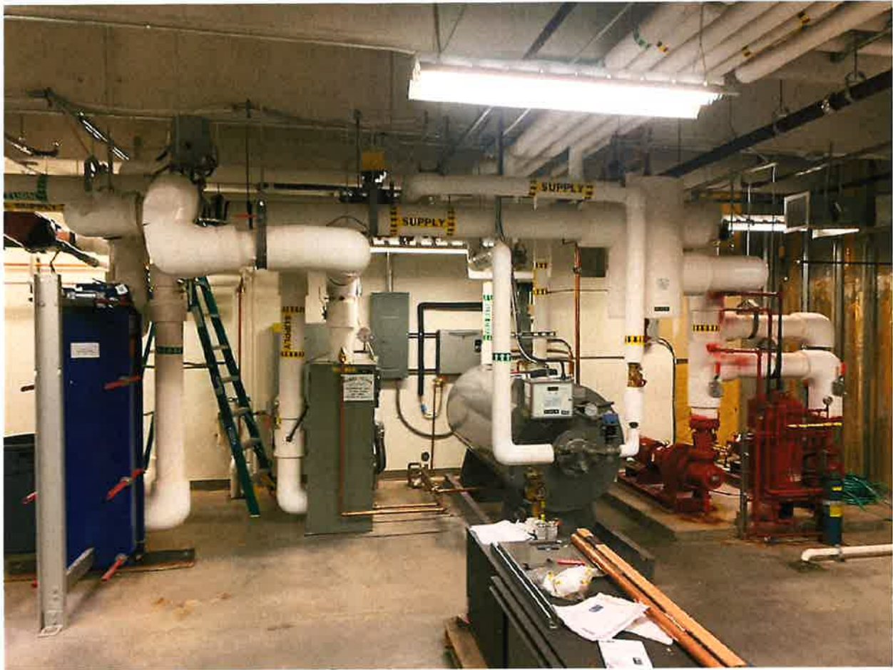
Main heat exchanger room in the basement of the Colter Building. The two motors are red in the bottom right corner.
