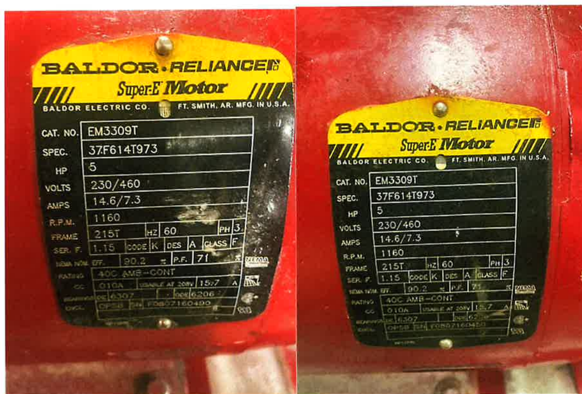
The two 5 hp motor nameplates
