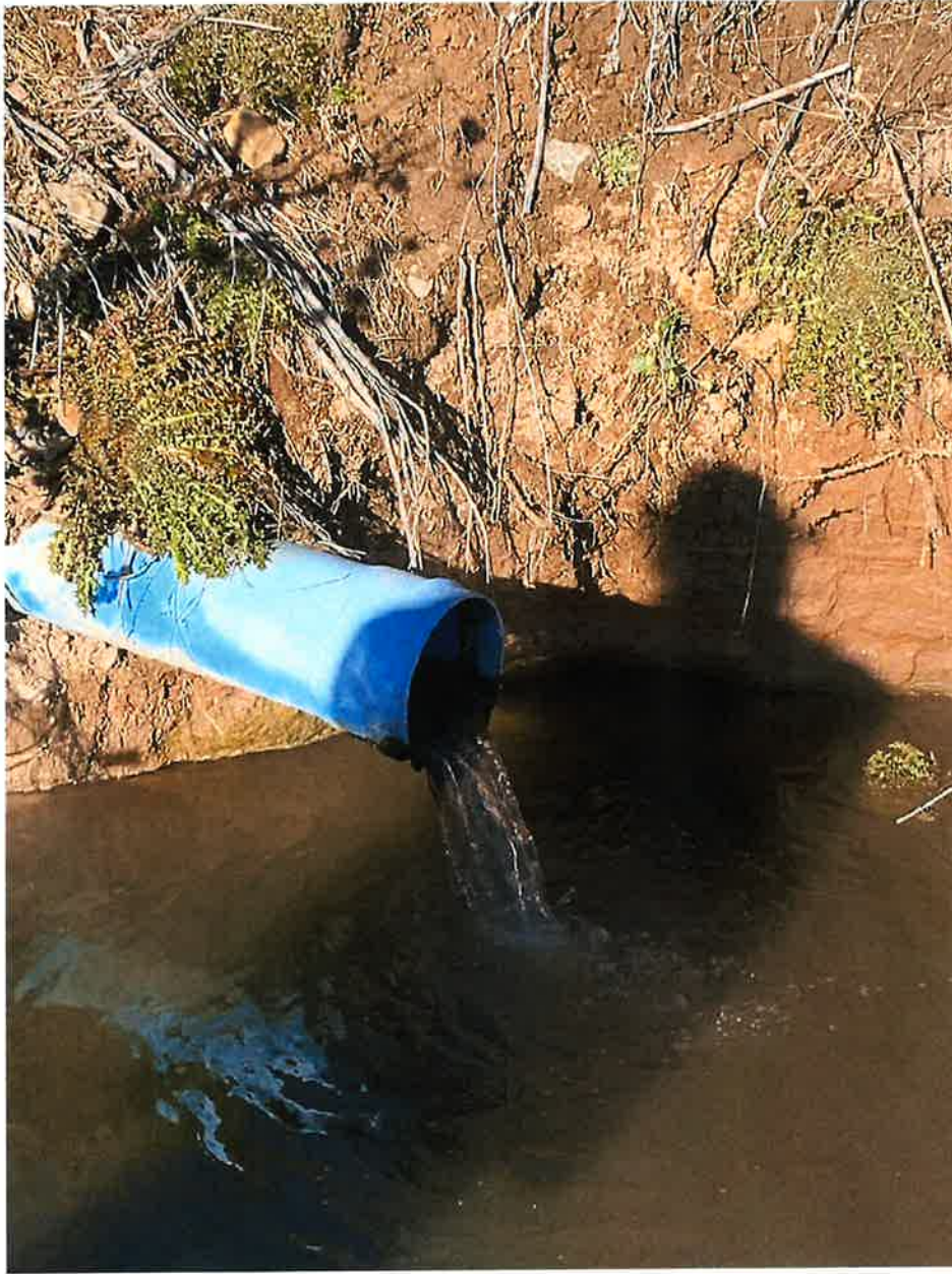
10" Horizontal Pipe Discharging Indoor Hatchery Water into pond @ 1.5 inches depth
