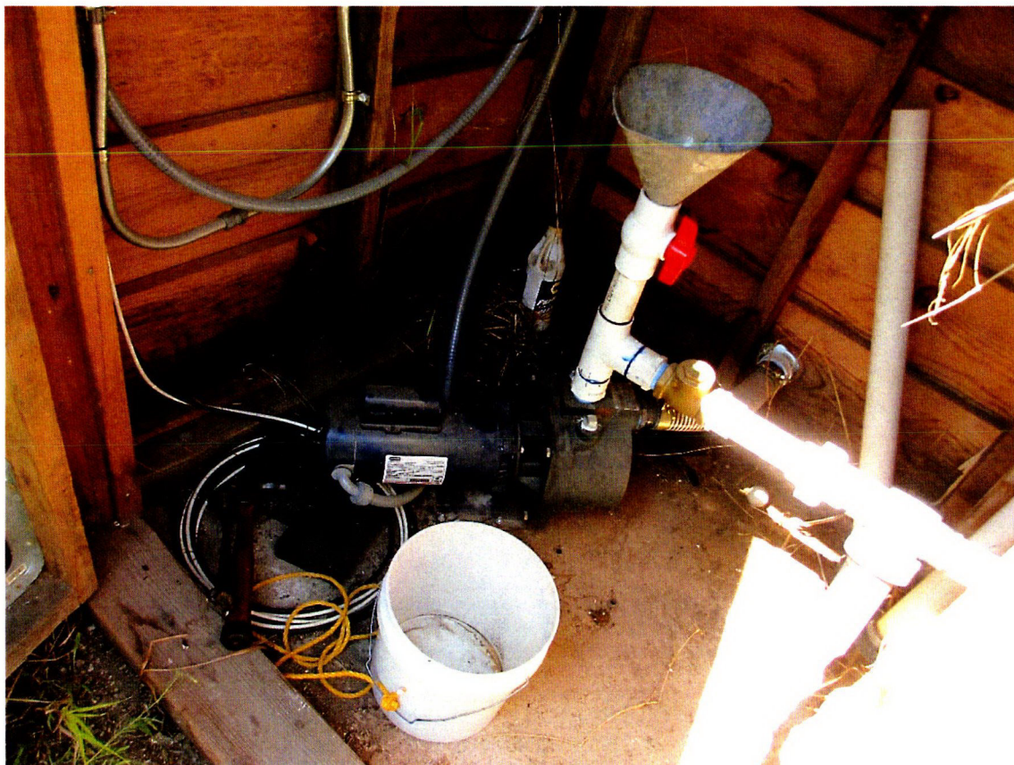
Pump and plumbing in pump house
