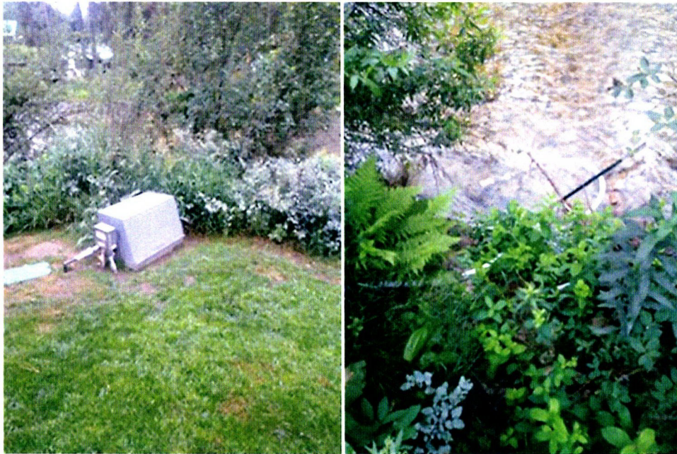
Photo 5 & 6- Pump and control box are in the left image and the screened intake is visible in the right image.
