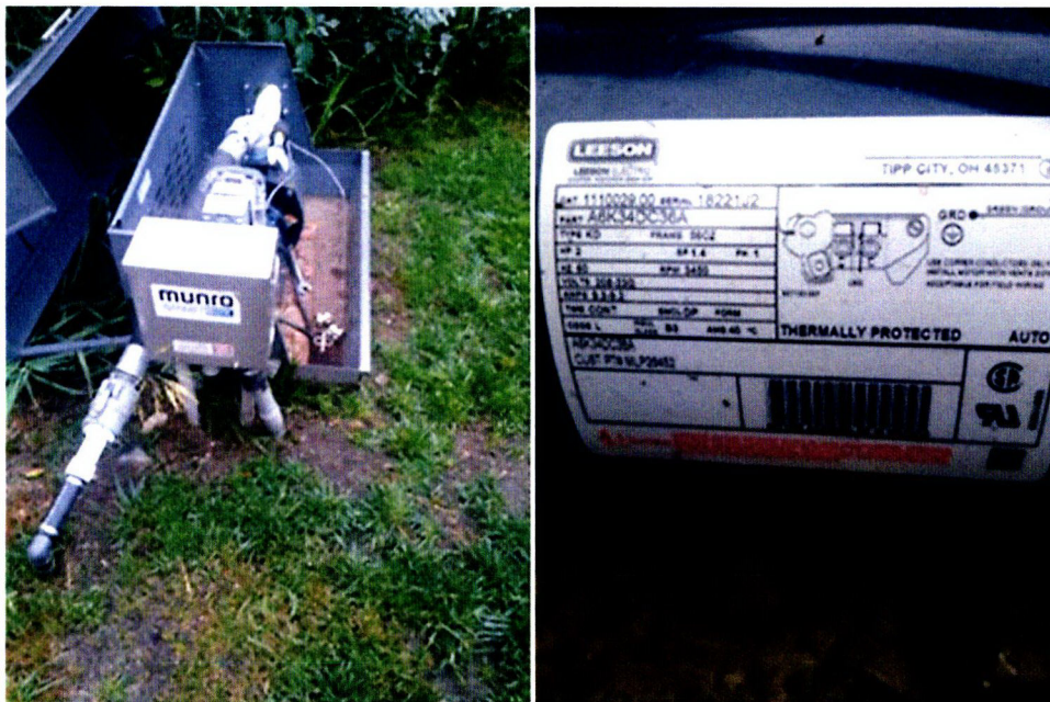
Photos 7 & 8- Pump with 2.5 Hp Leeson motor.
