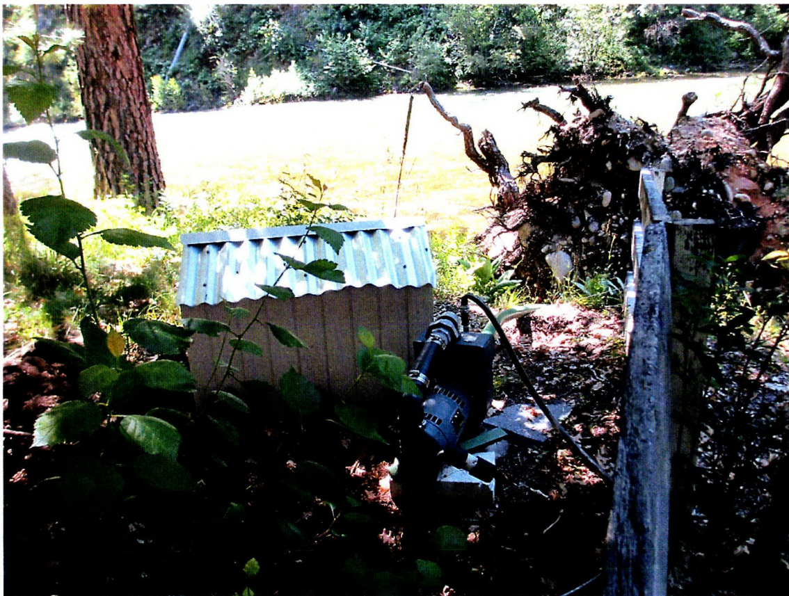
Pump with hose leading to river and irrigation line to lawn and landscaping
