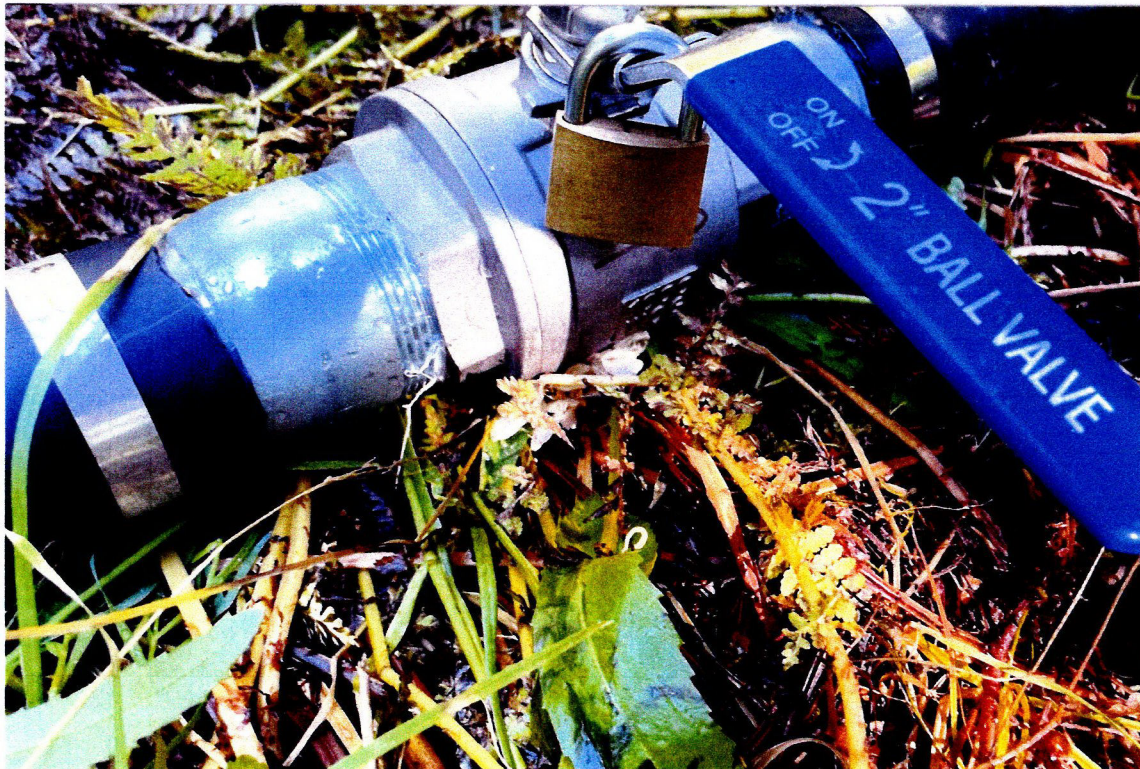
Lower diversion- Locking 2" ball valve in closed position
