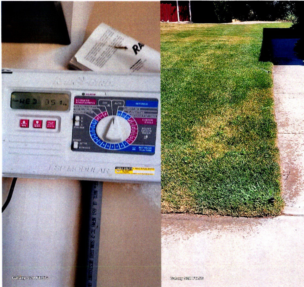
Photos 1 & 2- From left to right. The control panel for the home Rainbird sprinkler system with 9 zones. Photo 2, Umbrella sprinklers used around the home in the lawn.
