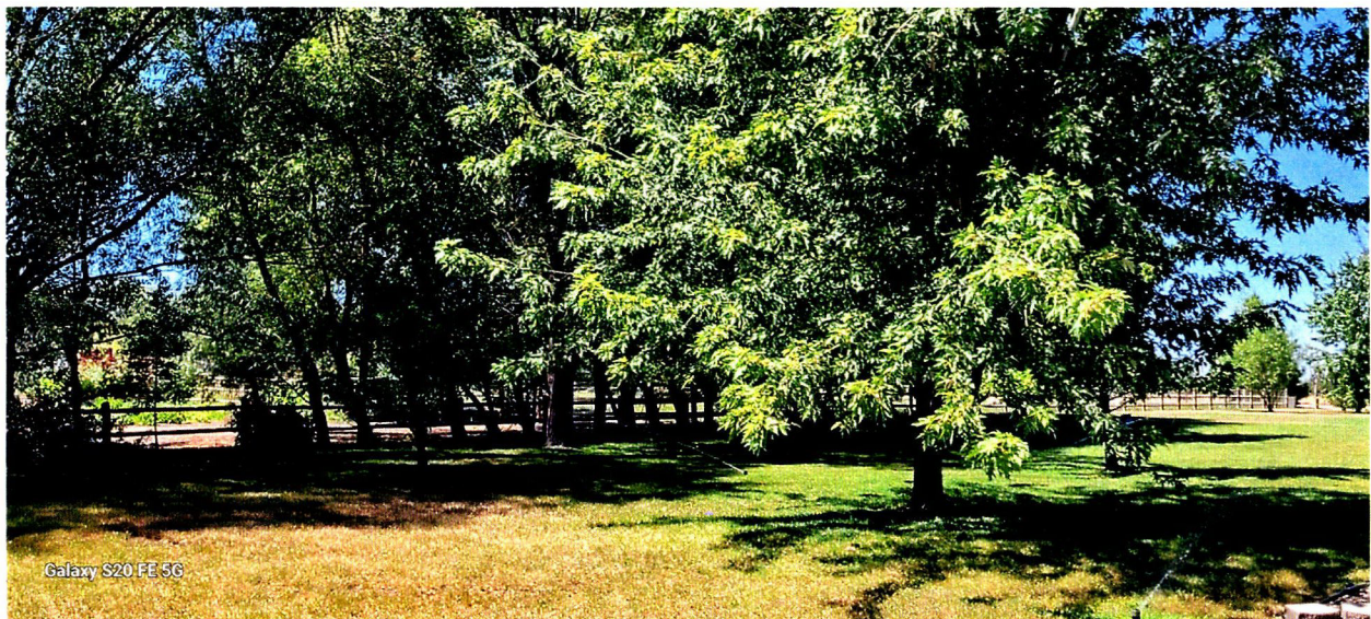
Photo 3- Home System-Rainbird rotary sprinklers, in the trees on the west side and back of the home.
