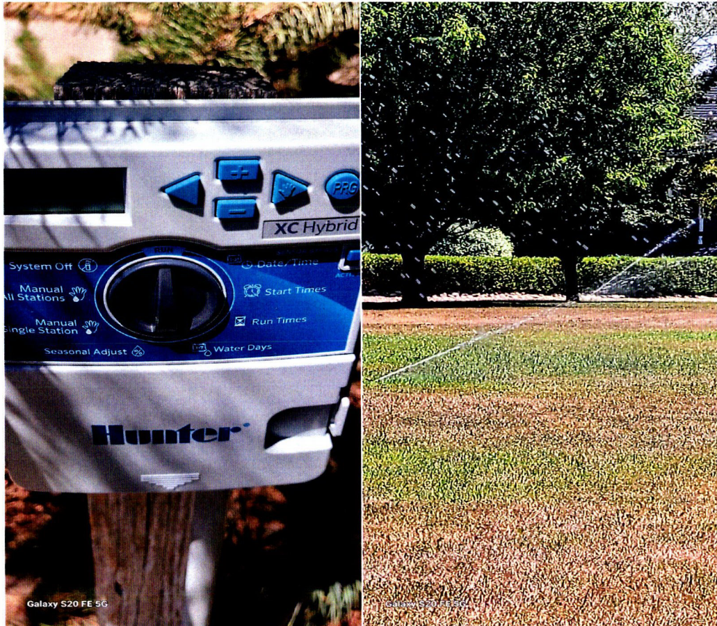
Photos 4 & 5- From left to right. Control panel for the Hunter sprinkler system (5 zones) on norther property and up to the roadway. Photo 5- Hunter rotary sprinklers used to water north side of property up to the roadway.
