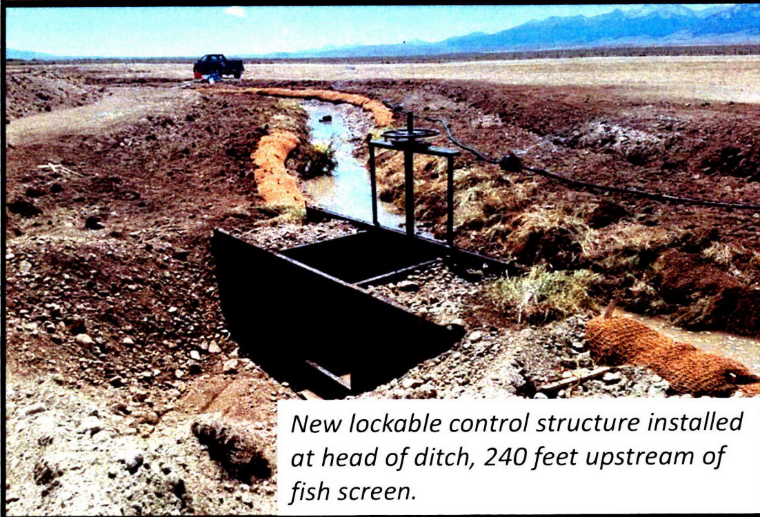
Fish screen with bypass pipe flow (.80 cfs) returning to Eighteenmile Creek.
