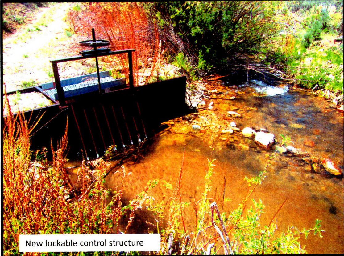
Fish screen with bypass pipe flow (.80 cfs) returning to Canyon Creek.
