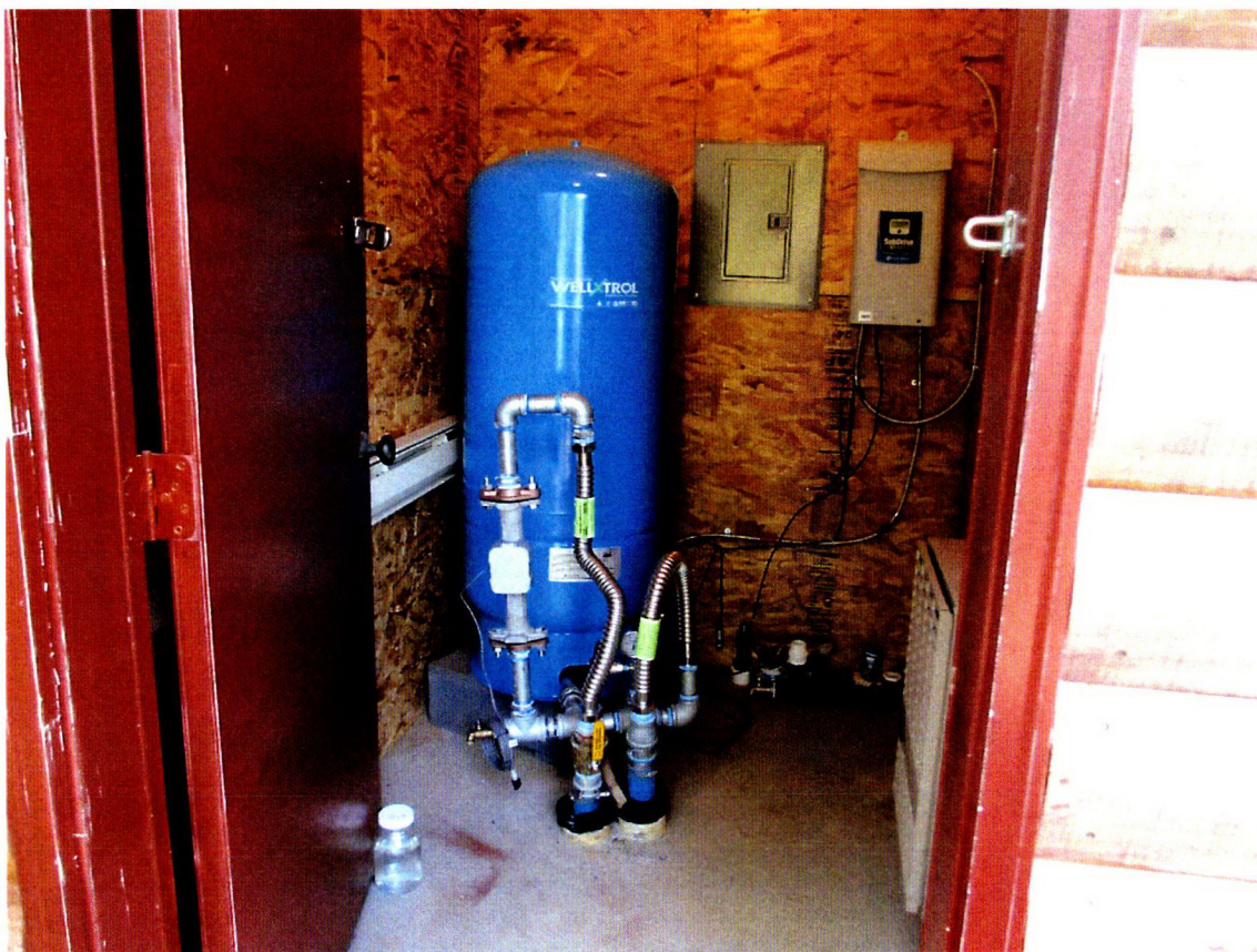
Plumbing inside pump house
