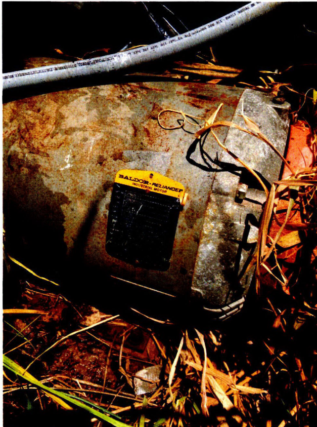
Fig. 5 – One 25 hp motor directly connected to the uphill 8" mainline pipe.
