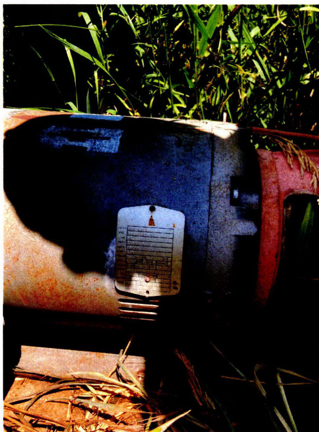
Fig. 6 – One 25 hp motor directly under the pipe cross fitting.
