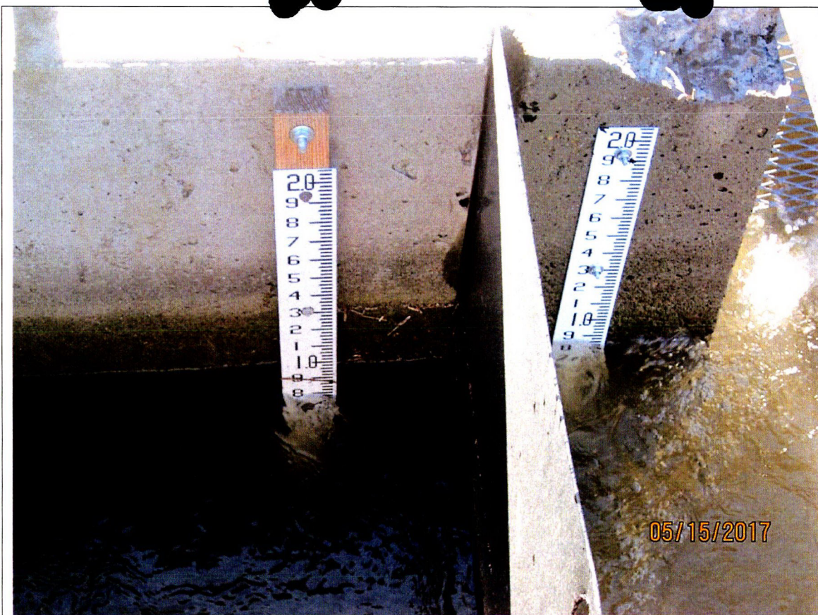
Figure 3. Staff gages on either side of headgate.
