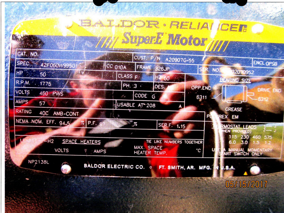
Figure 7. Specifications tag on motor.
