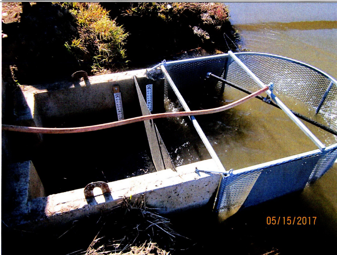
Figure 2. Trash screen and headgate box for POD.
