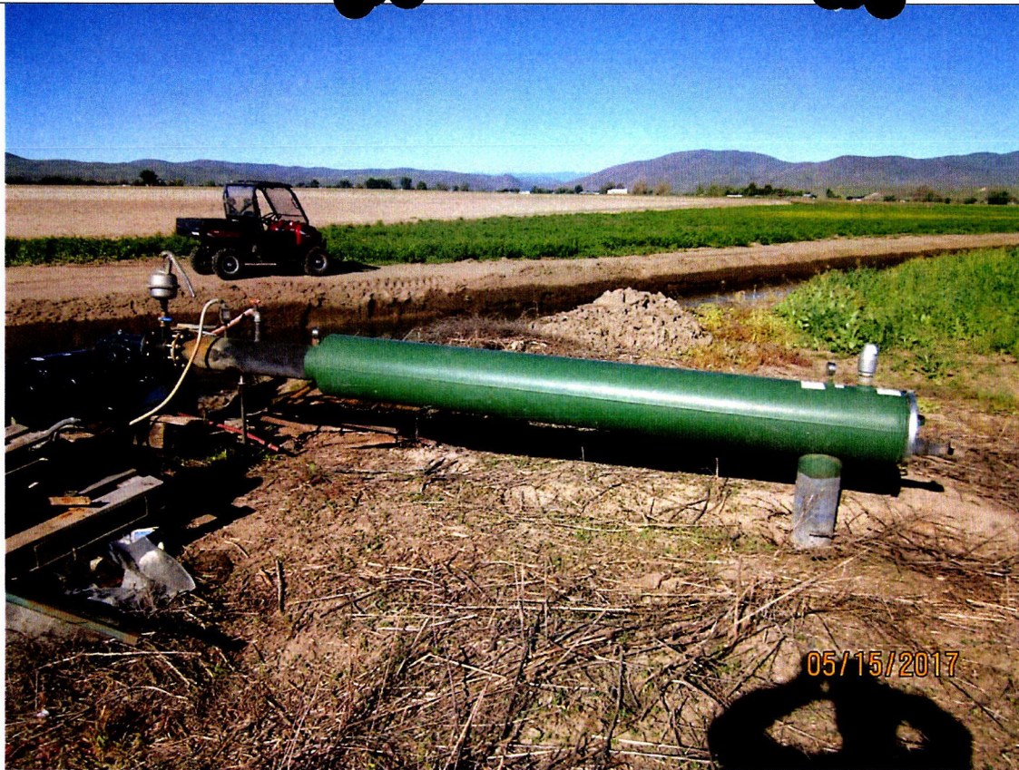
Figure 5. Location of pressure gage along filter.
