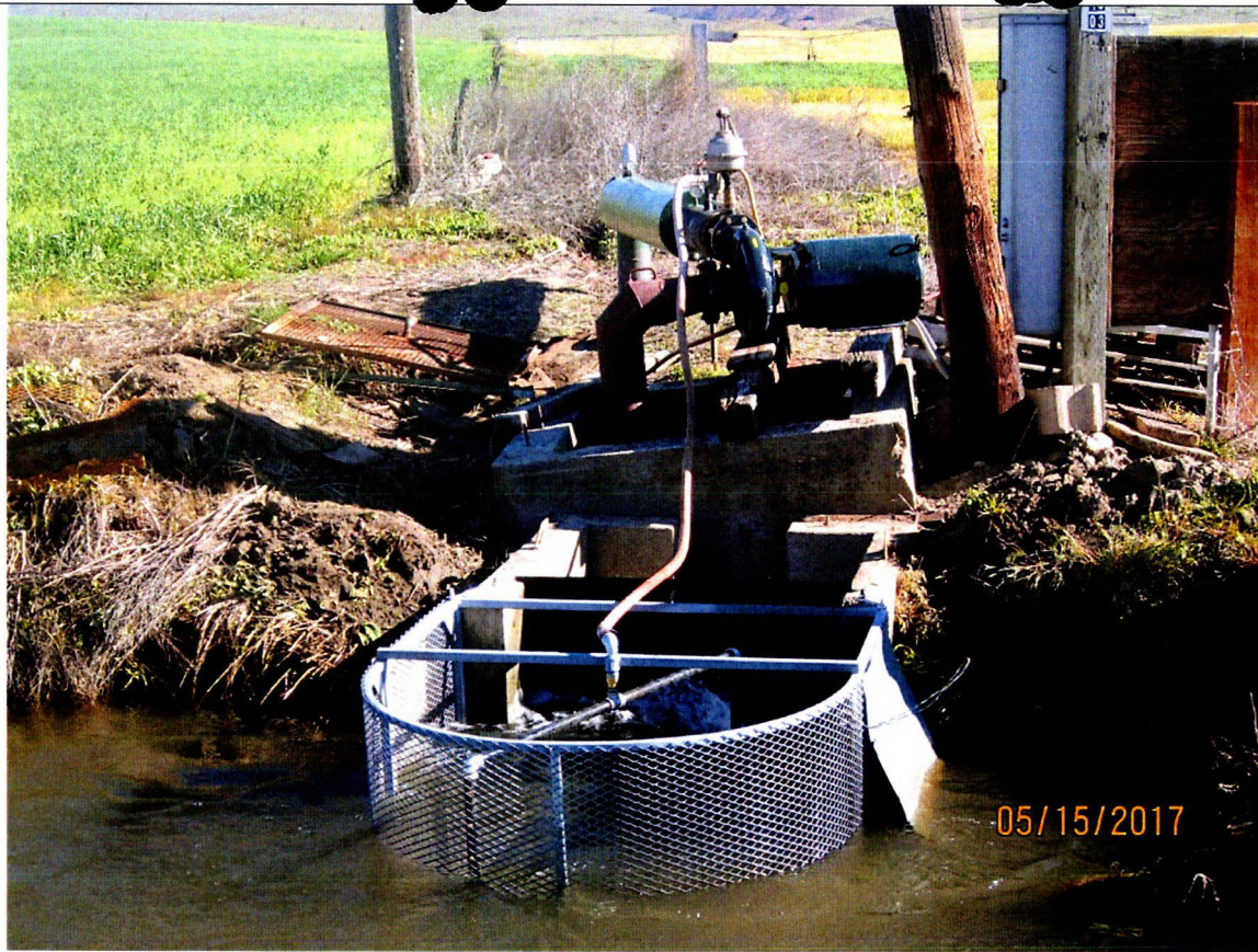
Figure 1. Pumping station for WR 67-15135 on the bank of the Galloway Canal from the Weiser River. The red pipe is 4.5 ft total long, and 2ft is submerged in the water.
