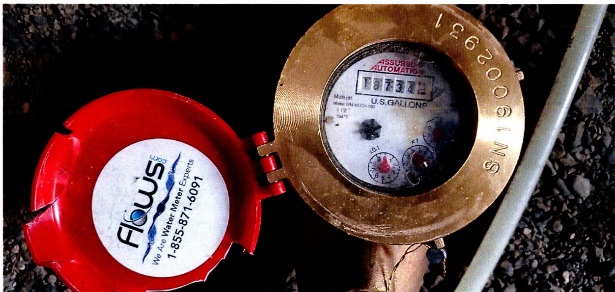
Figure 6: Close up of the meter at the well
