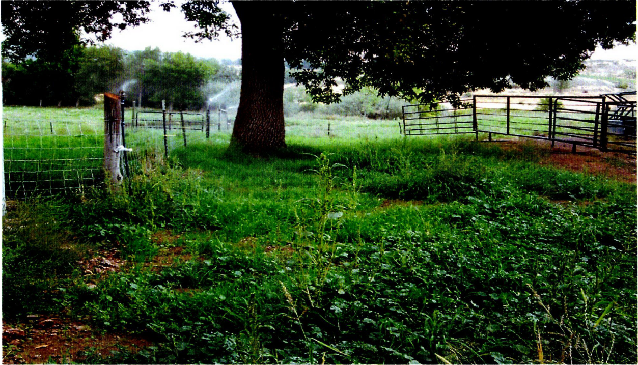
Above: Sprinkler system, northeast side and middle
