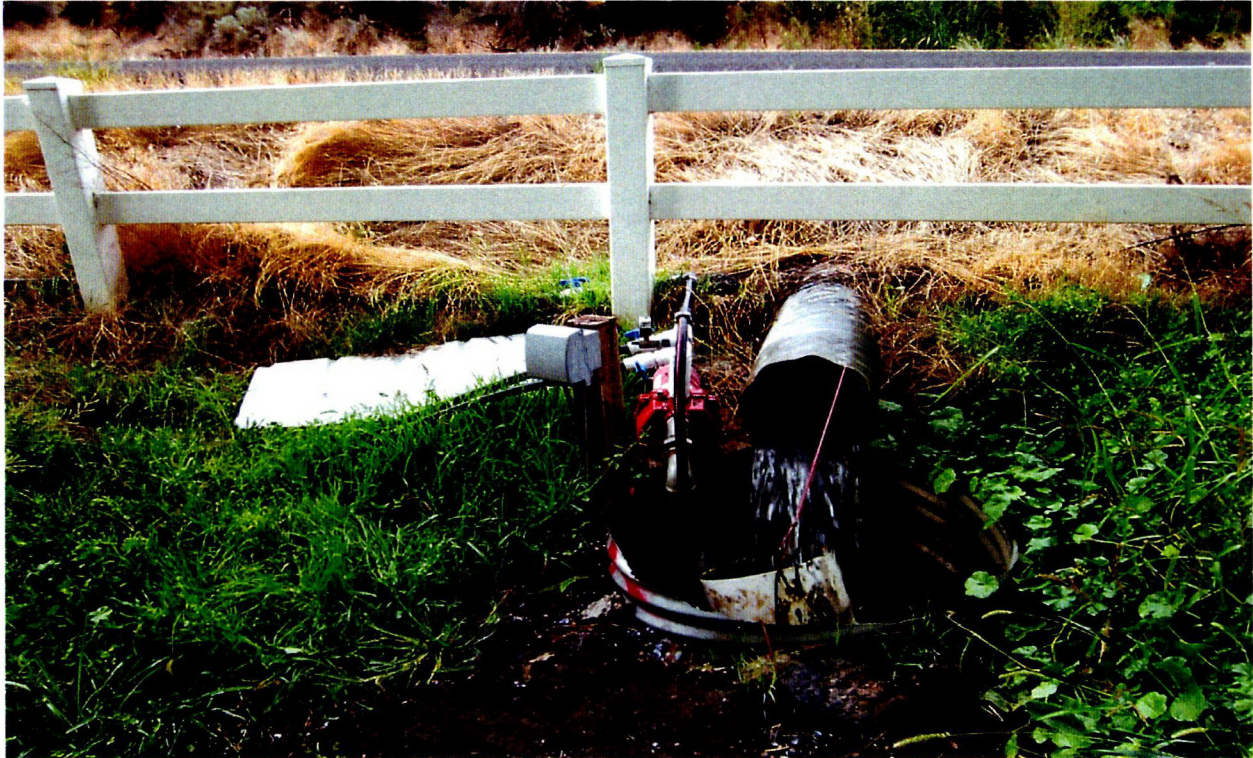
Above: Waste water from neighboring farms into standpipe, where water is pumped into sprinkler system
