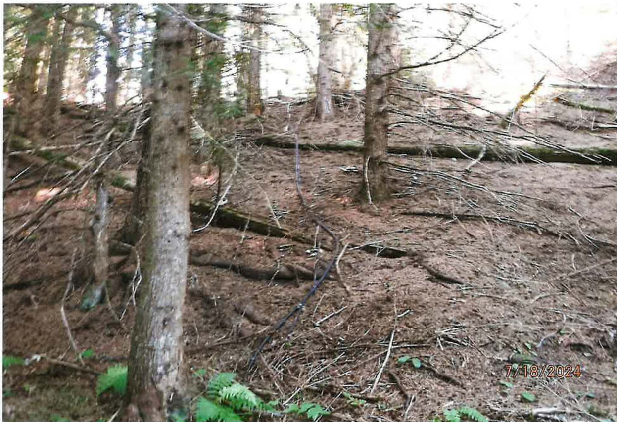
¾-INCH CONVEYANCE POLY PIPELINE FROM POD UP-SLOPE TO 1,000-GAL STORAGE TANK
