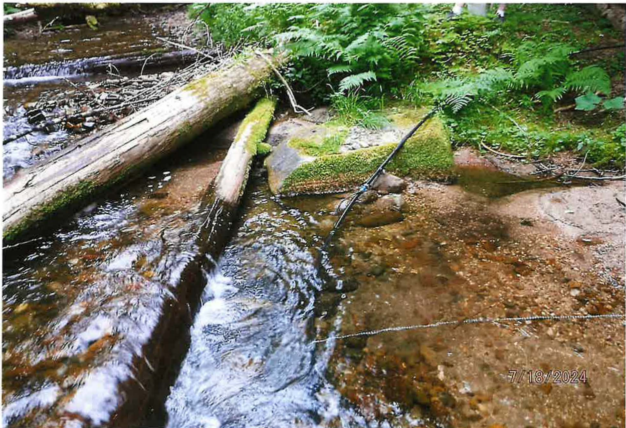
POD – SUBMERSIBLE PUMP IN CREEK
