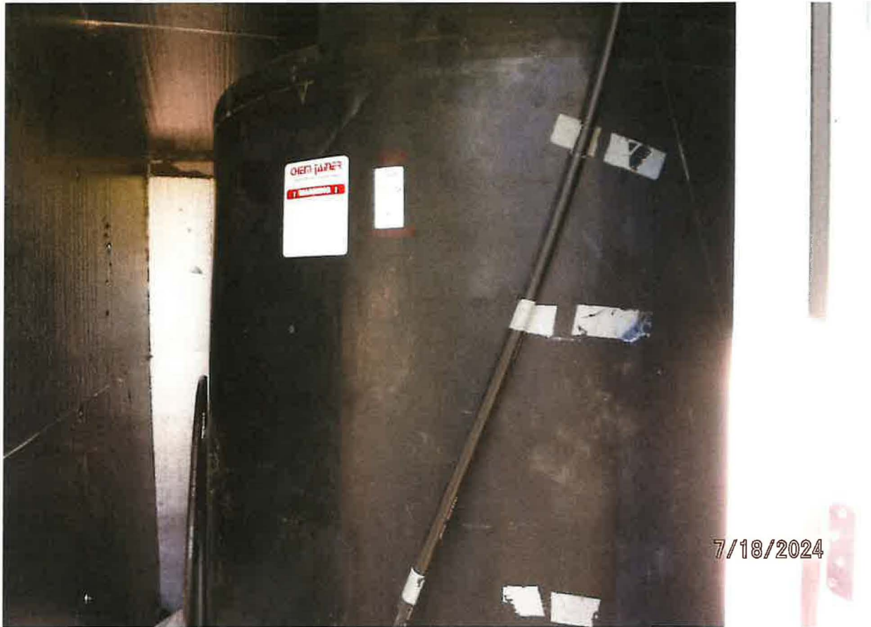
1000-GAL STORAGE TANK TEMPORARILY STORES WATER FOR STOCKWATER AND IRRIGATION USES
