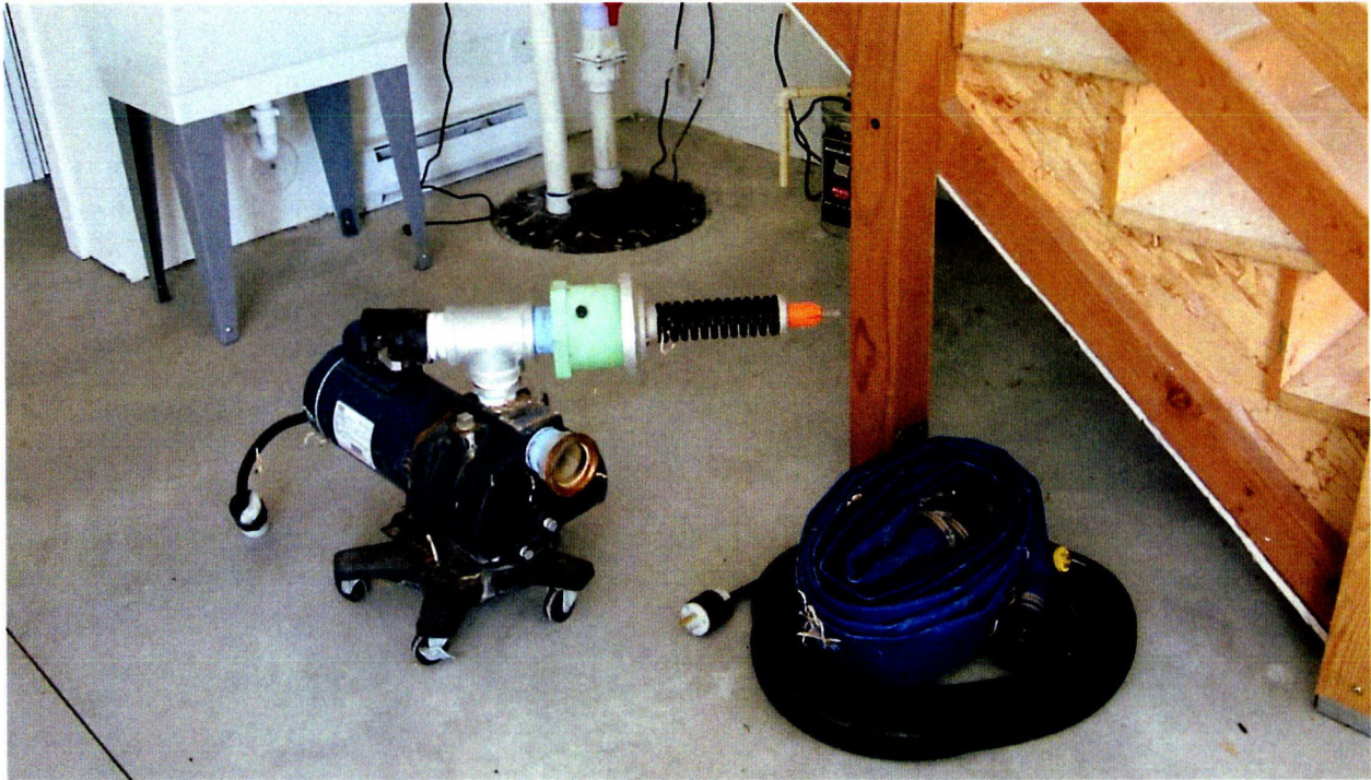
Electric Power Cord, Pump, and Hose for the irrigation system
