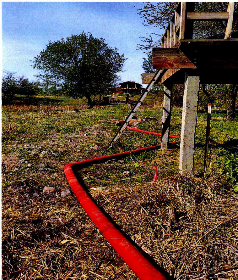
Fig. 4 - Picture of 4' Camlock hose from pump tying into 4" PVC pipe that leads towards house 250 feet in T01N 03W section 8 SWSE SE NW QQ. Facing West.
