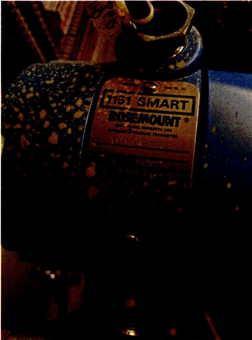
Turbine 1 Meter: Meter records flow rate for Turbine 1. Serial No. 0987246.
