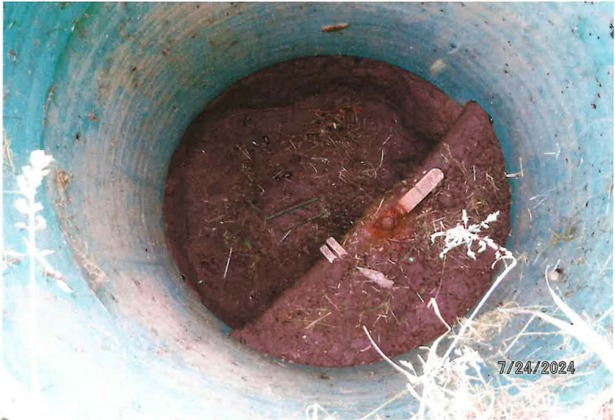
MAIN WATER LINE SHUTOFF VALVE LOCATED BETWEEN PUMP HOUSE AND 1 ST RESIDENCE ON SYSTEM
