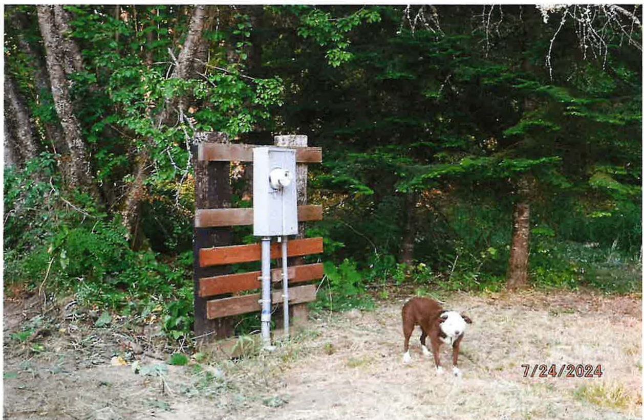
SEPARATE POWER SYSTEM SERVES THE SPRING SOURCE WATER SYSTEM THAN REST OF 4 EA HOME(S) POWER ELECTRICAL GRID
