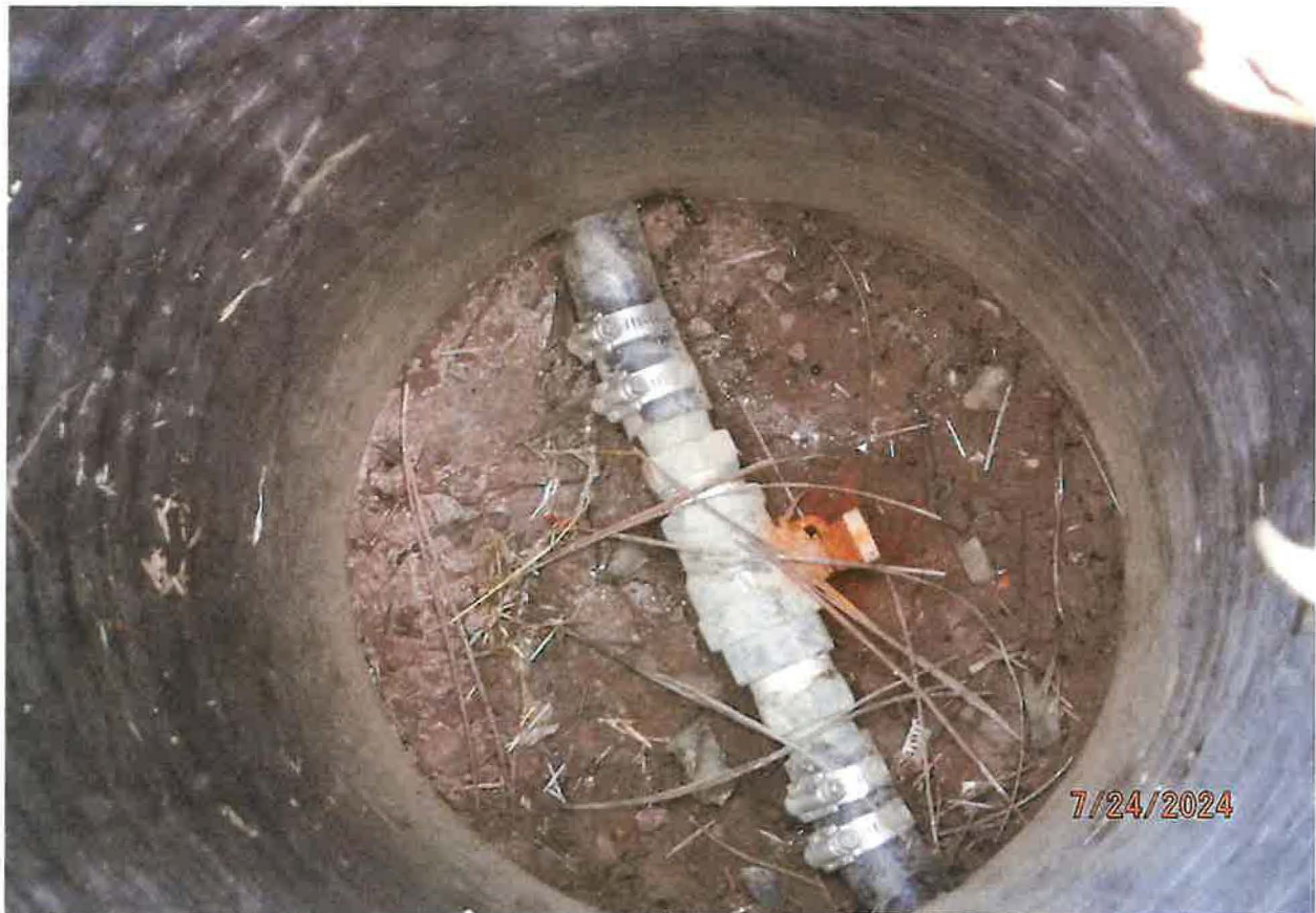
MANUAL SHUTOFF VALVE FOR 4 TH HOME – HOME IS CURRENTLY IN CONSTRUCTION BUT WATER IS SERVICE CONNECTED TO RESIDENCE AND IN USE ON THE PARCEL
