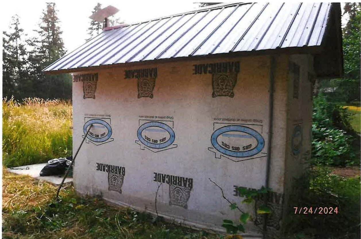
SPRING GRAVITY FLOWS IN 1 ½ INCH POLY PIPE TO 2,400 GALLON VAULTED RESERVOIR
