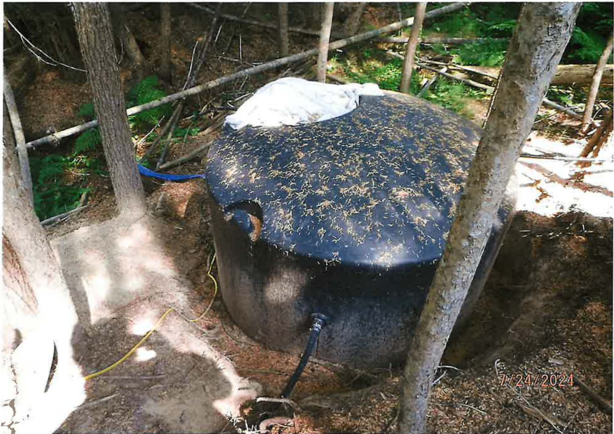
½-INCH PIPE INFLOW TO 635- GALLON STORAGE TANK, WHICH USES A 1-HP PUMP AND PIPELINE CONVEYANCE SYSTEM TO DISTRIBUTE STREAM WATER FOR BENEFICIAL USES
