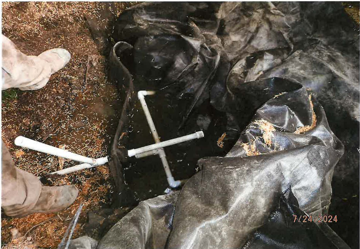
POD – UNNAMED STREAM CAPTURED IN POOLING WITH ½-INCH PVC PIPE DRILLED WITH ¼-INCH HOLES GRAVITY FLOWING TO STORAGE TANK
